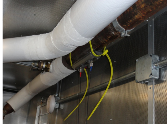
Ultrasonic Flowmeter Verification of FL1
