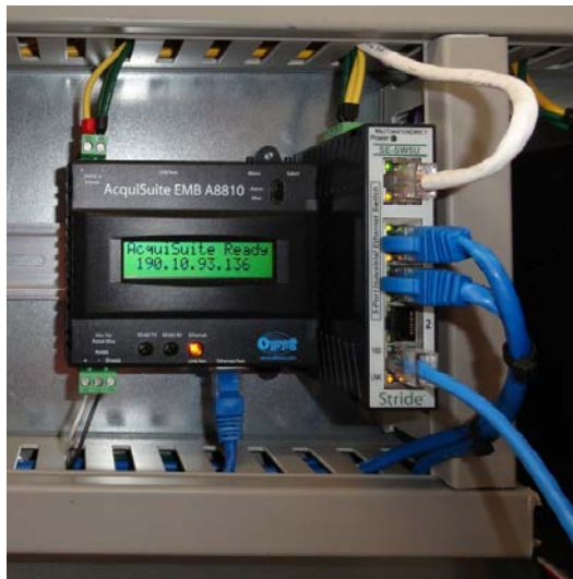
Figure 2. Data Logger Installation
