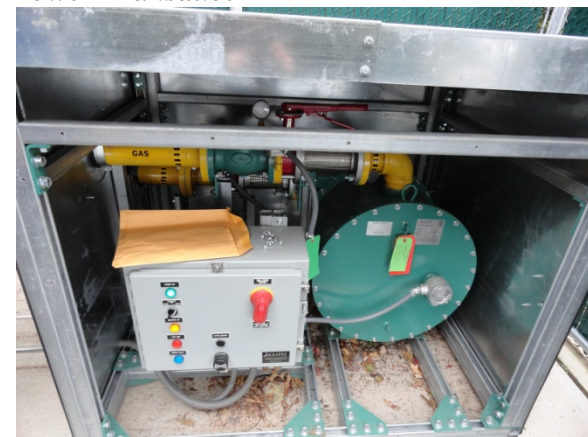
Gas Booster Compressor (430 W added to WPAR)
