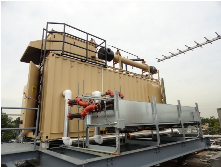
CHP Container and Dump Radiator On Rooftop
