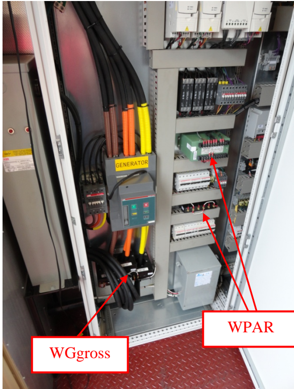
Generator Disconnect and CTs, Parasitic Power Transducer
