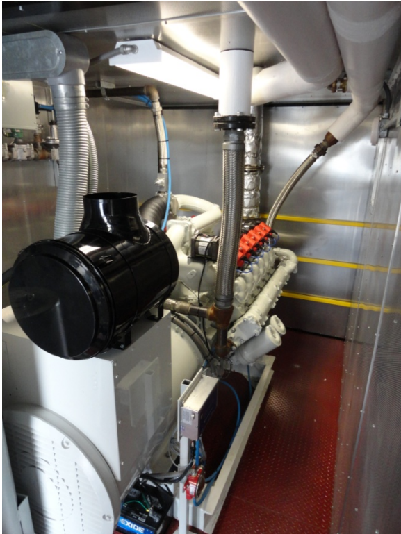
Mann 250 kW Engine Generator
