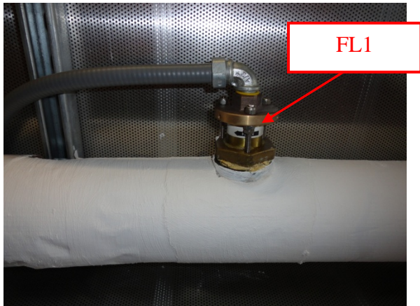
Primary Loop Flowmeter
