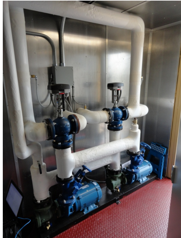
Engine Loop Pumps, Building Loop Valves (Right) and Radiator Valves (Left)
