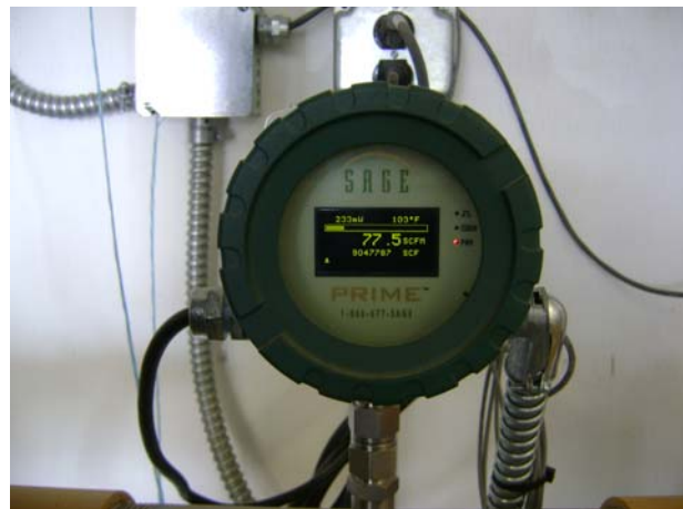
FGE – Sage flowmeter measuring biogas to engine.
