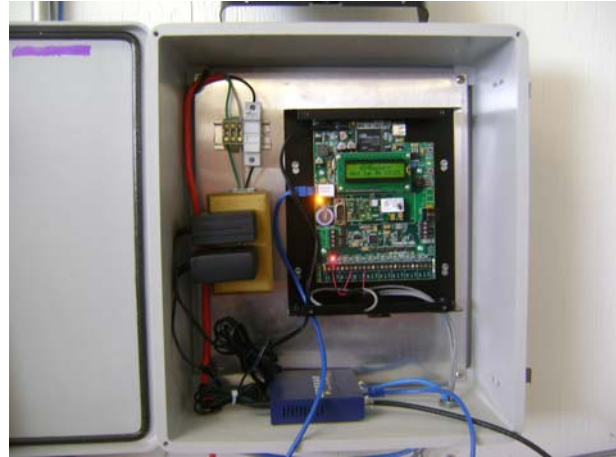
Interior of CDH enclosure – Obvius AcquiSuite data logger.
