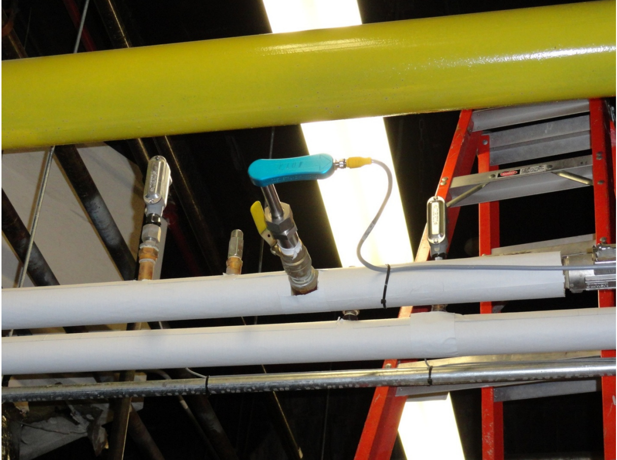
TLS2, TLR3, FL2 Location on Boiler Loop Piping (Overhead)
