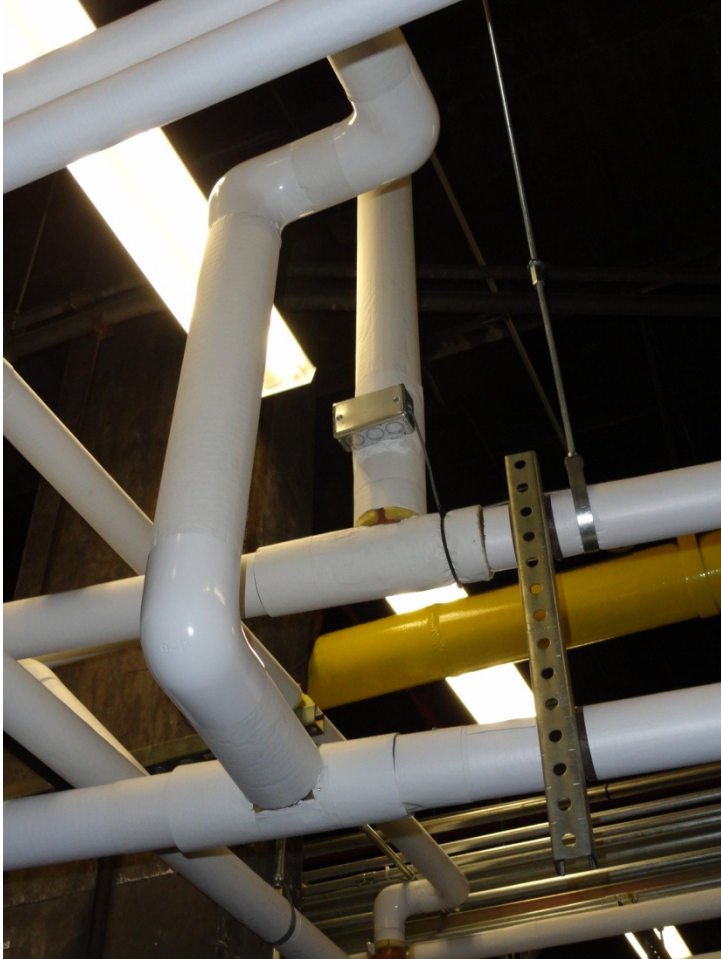
TLR2 Location (Overhead) Returning from Dump HX (Above Roof)
