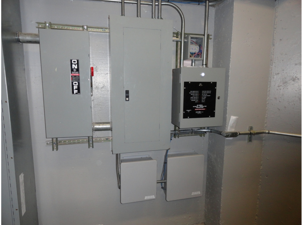
Data Logger and Power Transducer Panel Location
