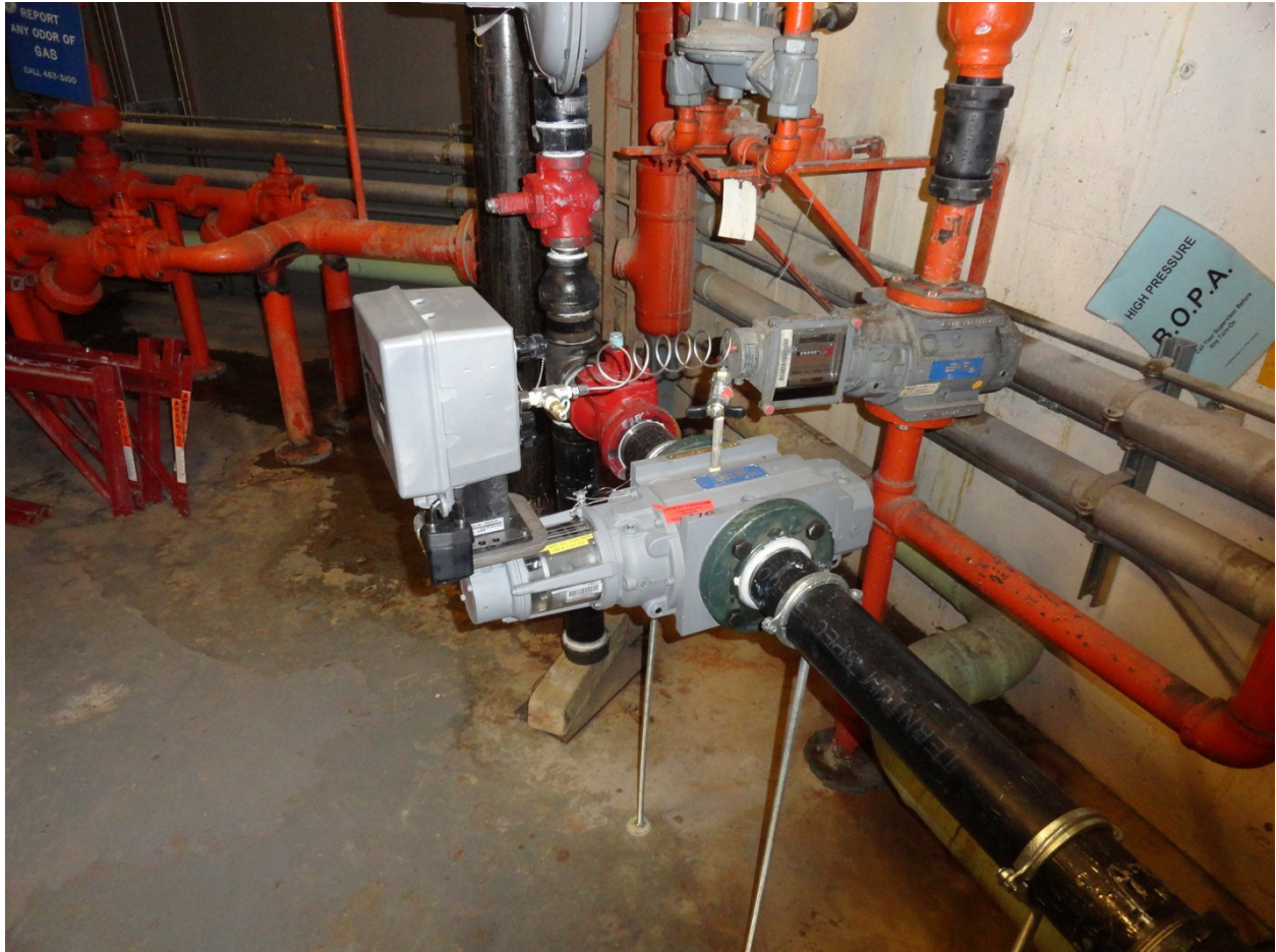
Gas Meter (No Pulse Output as of 2012 July 12)
