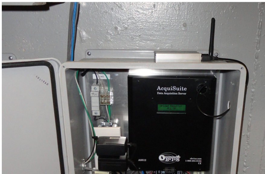
Cellular Modem on Top of Data Logger Panel in Boiler Room
