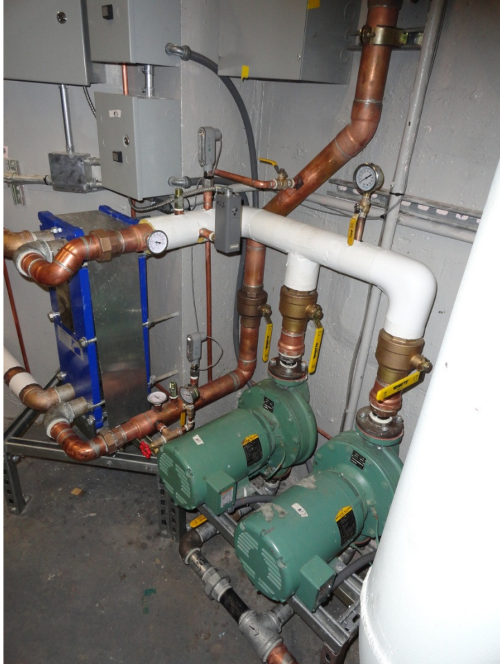
HX 1 and TLS1, TLR1 Location on DHW Loop Piping
