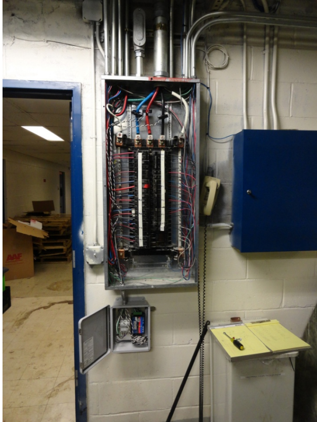
Parasitic Load Panel EPP-C-1 and Power Transducer (WPAR)
