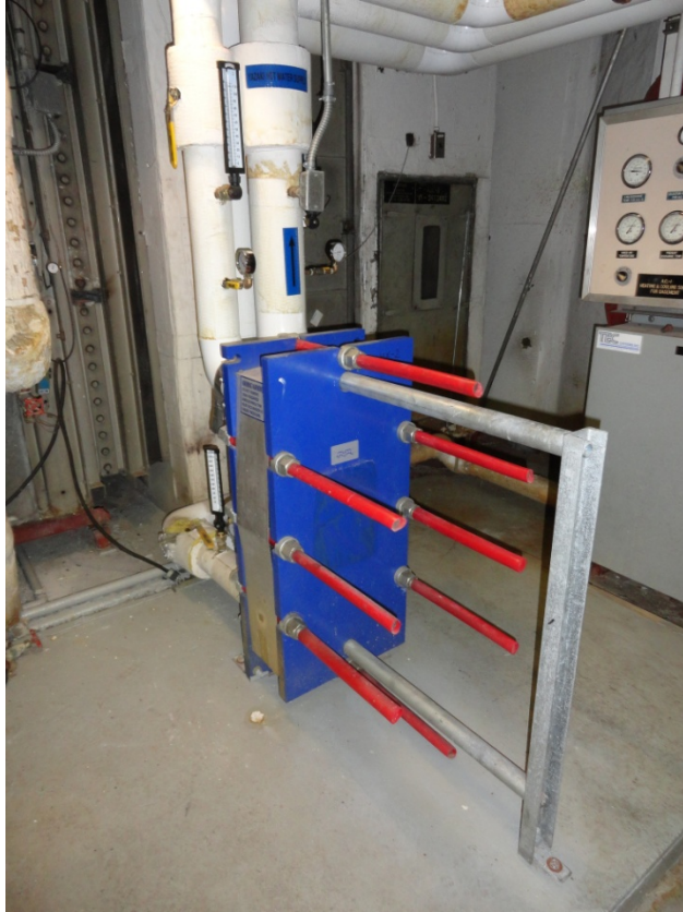
HX2 – Absortion Chillers
