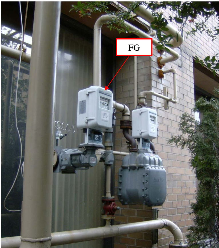
CHP Gas Meter (FG) – No Pulse Output Installed Yet
