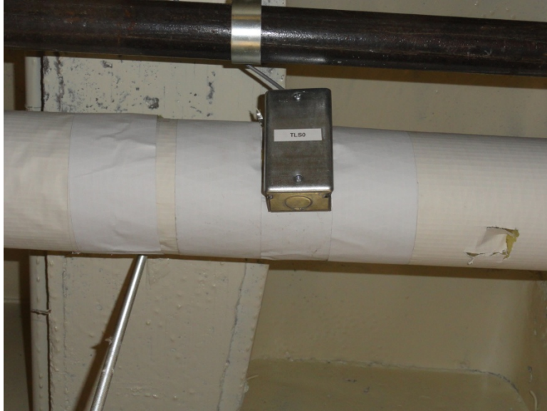
Heat Recovery Temperature Sensors ( TLS0 ) – Before Engine Chiller HX (Diagnostic) – In CHP Room
