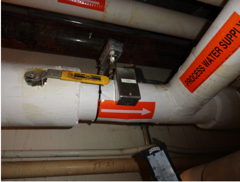
Heat Recovery Temperature Sensors (TLR2) – After Greenwall Space Heating HX (Diagnostic) – In Boiler Room
