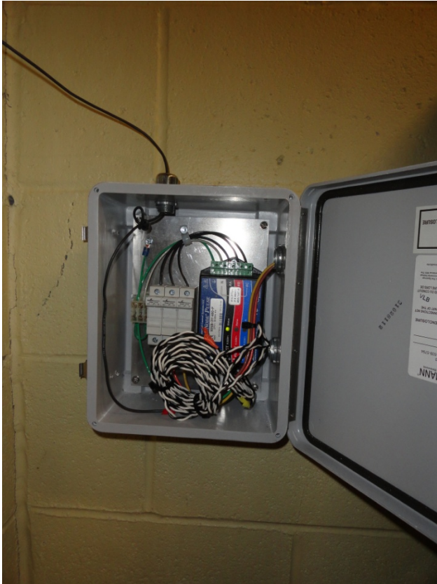
Generator Power Transducer (WG)
