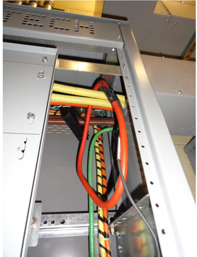
Generator Power Transducer (WG) Typical 600 A CT and Fluke Flexible CT for Verification
