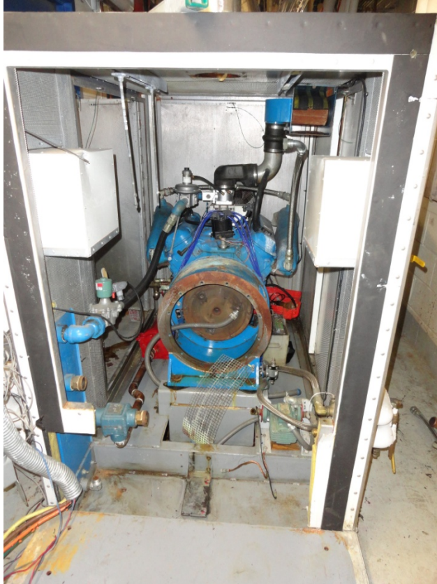
CHP Unit #3 – Inoperable – April 2012
