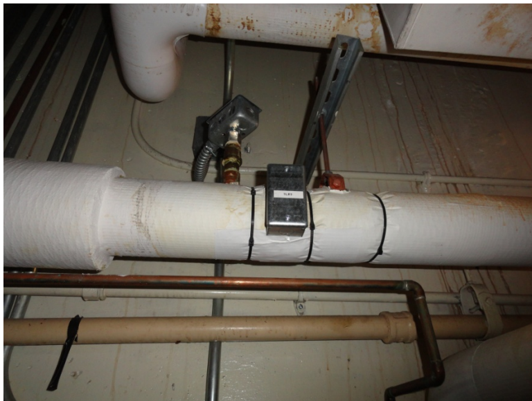
Heat Recovery Temperature Sensors ( TLR1 ) – After Absorption Chillers (Diagnostic) – In Boiler Room
