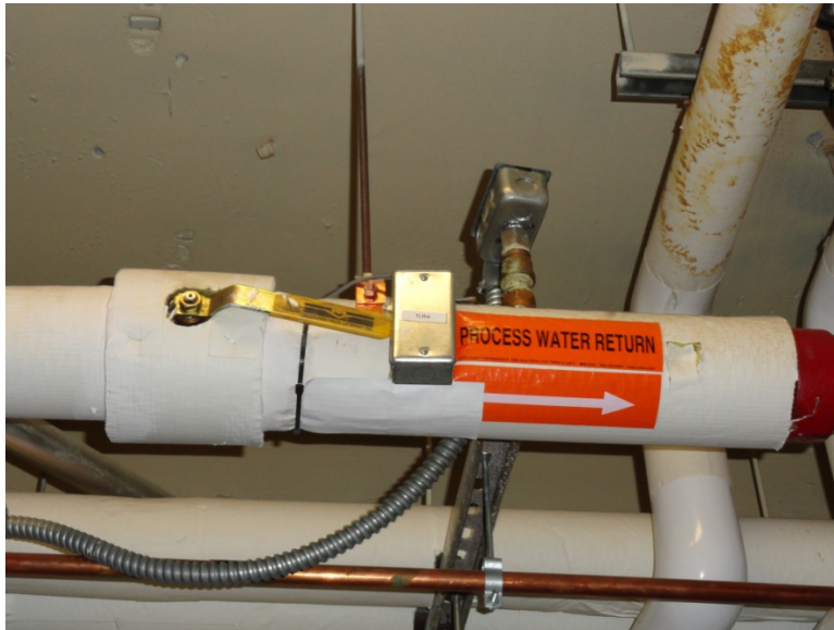
Heat Recovery Temperature Sensors (TLR4) – After Dump HX – In CHP Room
