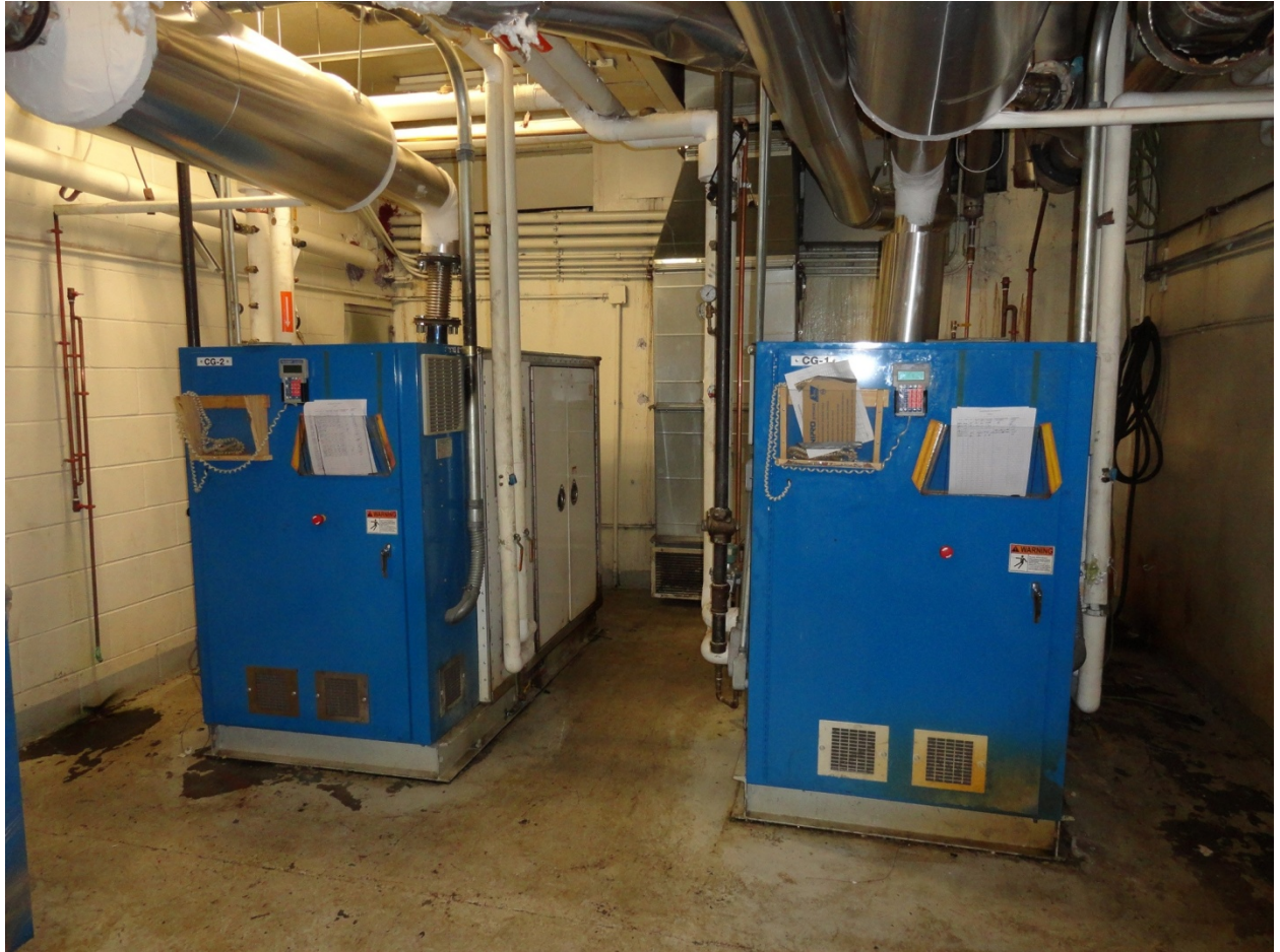
CHP Unit #1 and #2 (Operable)
