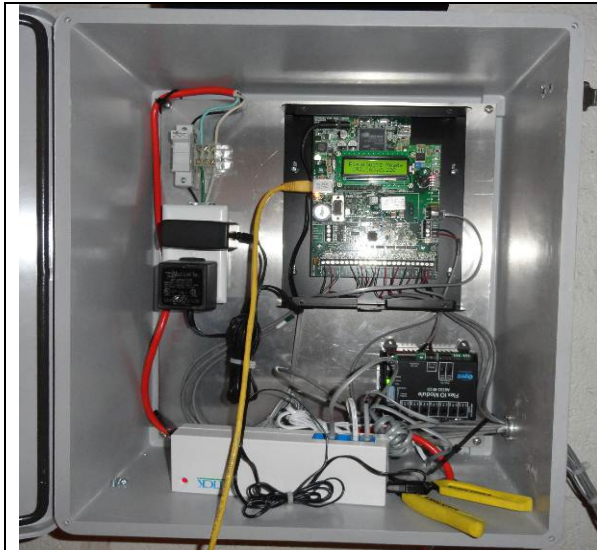
CDH enclosure and datalogger
