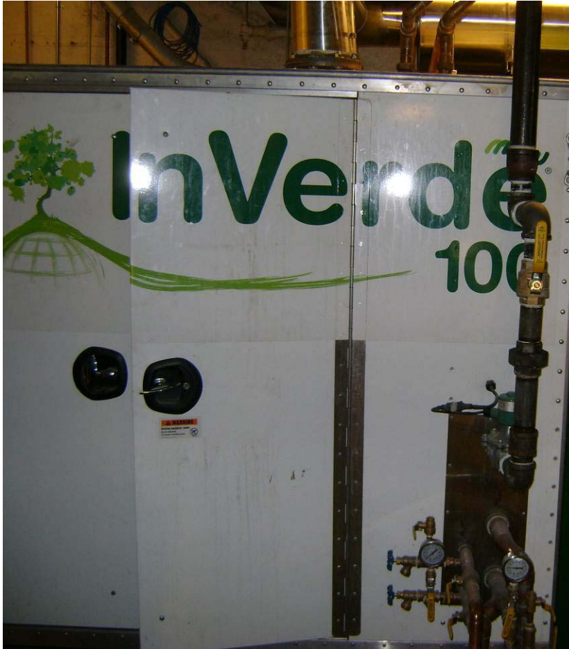
Figure 1. Photo of Tecogen InVerde 100 unit
