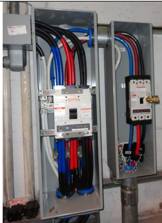
208 V disconnect (right) and CT's
