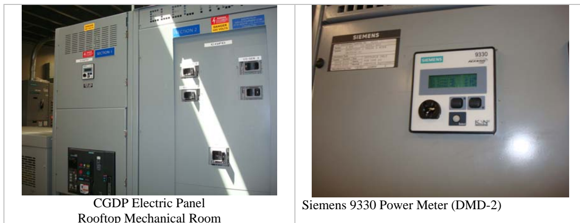
Figure 5. Power Meters for Generator Output and Total Facility Power
