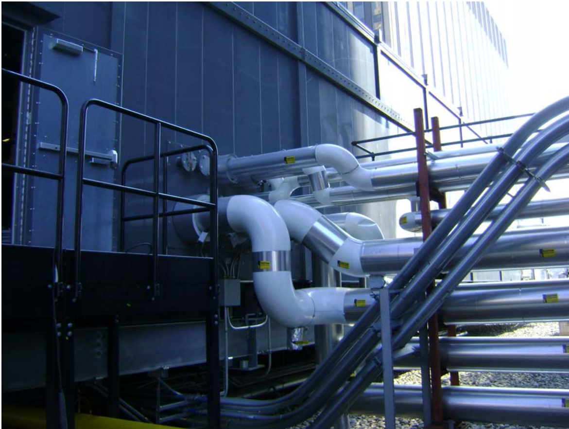
Connections to Cogen Enclosure (HW supply & return; CW supply & return; HP Steam out; LP Steam input; Condensate return; Makeup water)
