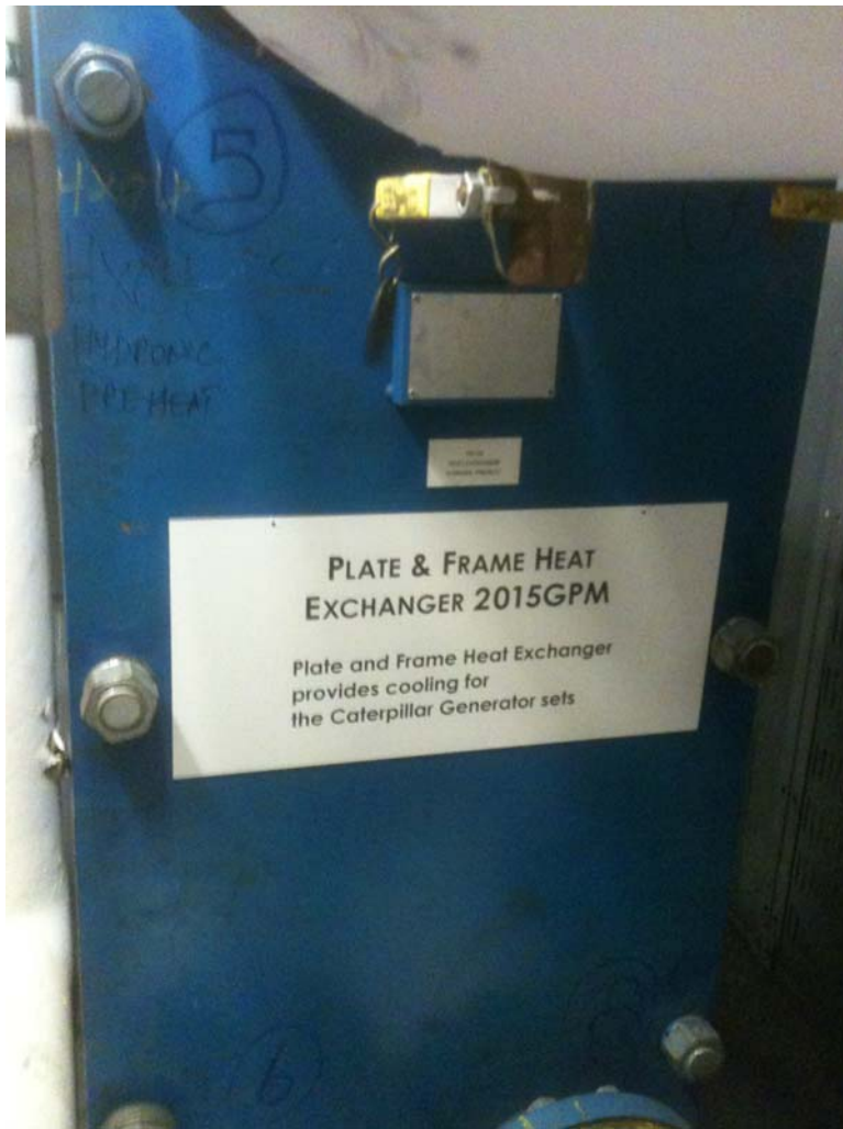
HX-04 (serves Perimeter Heating Loop)
