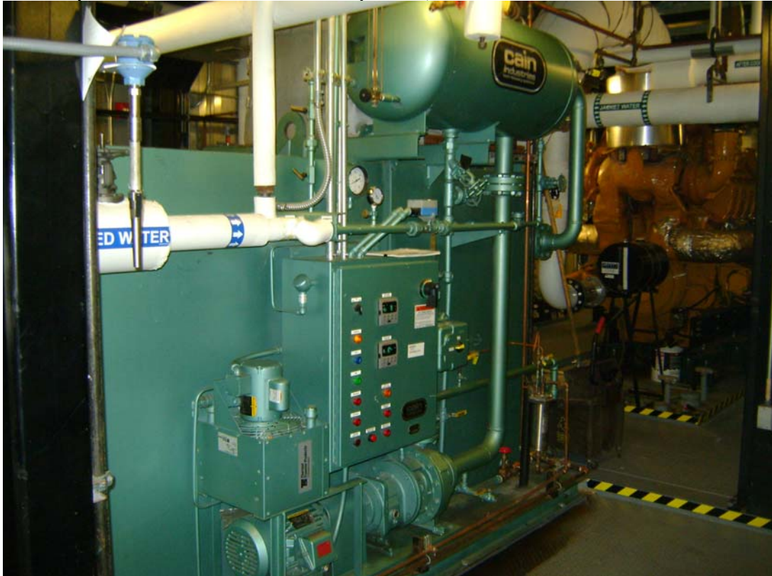
Cain Heat Recovery Steam Generator (1 of 3)
