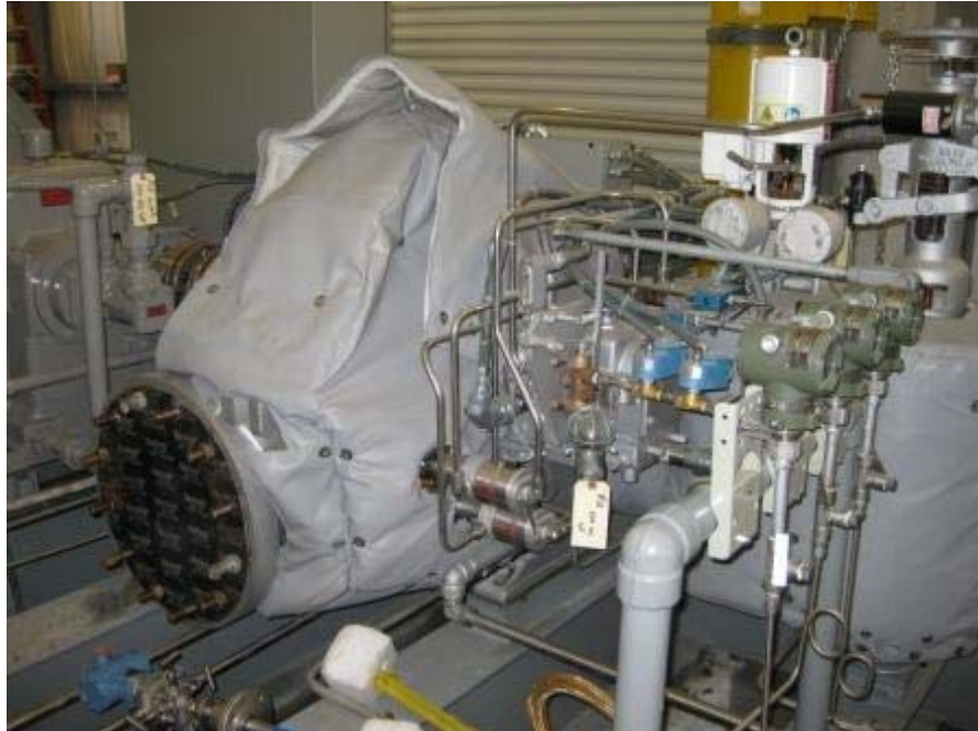
Fig 3: New Steam Turbine
