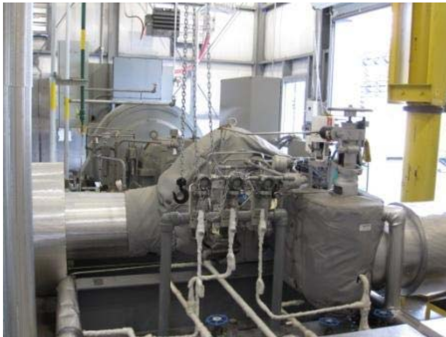
Fig 12: New Steam Turbine Generator
