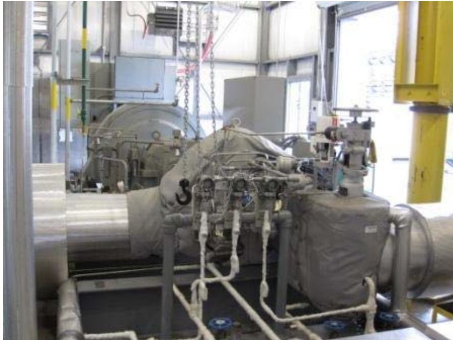
Fig 1: New Steam Turbine Generator
