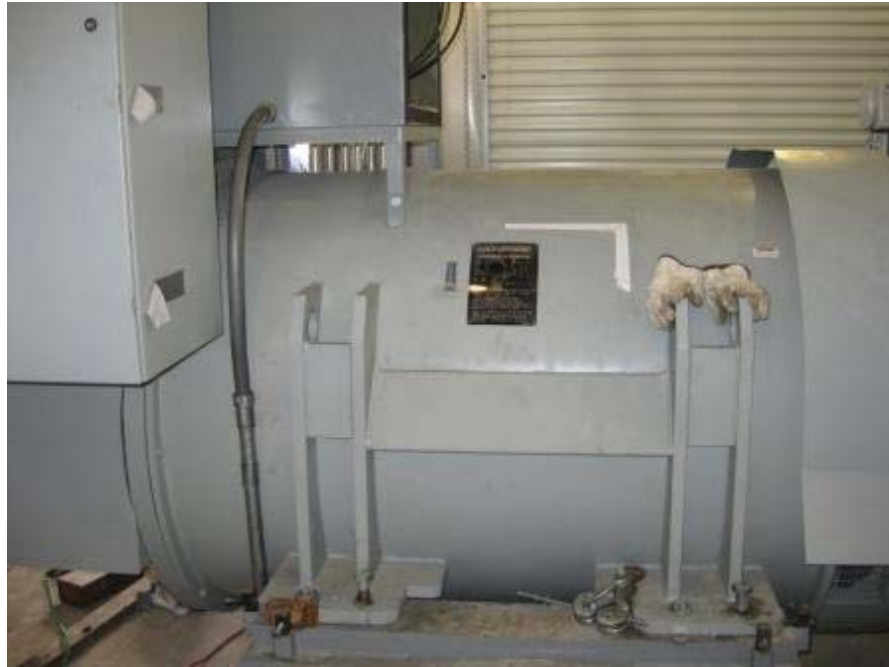
Fig 4: New 1 MW Generator
