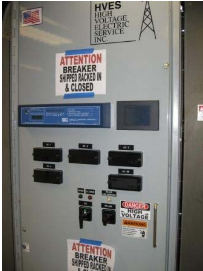
Fig 5: New Circuit Breaker
