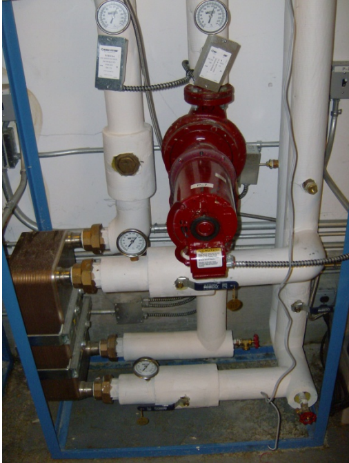
Dump Radiator Loop Pump P-7 and HX
