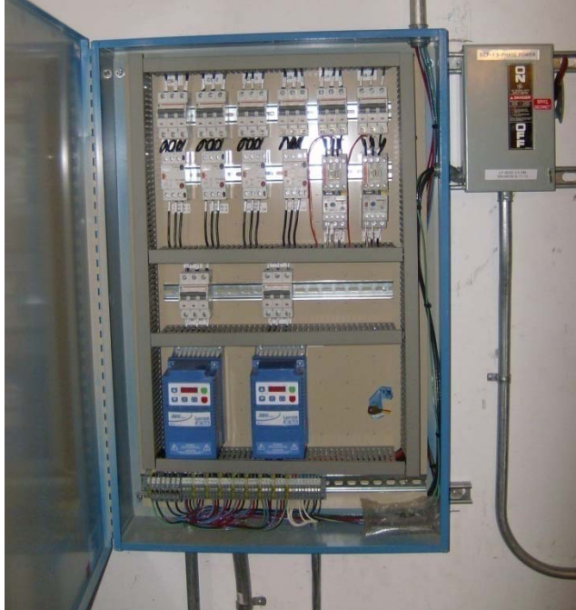
Figure 5. Parasitic Load Panel CCP-1
