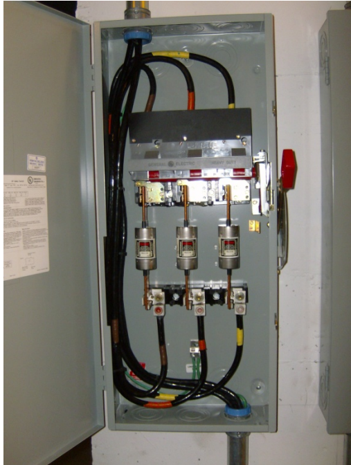
Figure 4. Engine Generator Disconnection Location of Power Transducer (1 of 2 typ)
