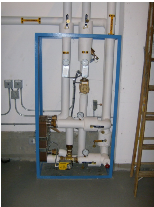
DHW Low Zone Pump (P-5) and HX
