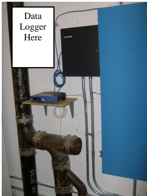
Data Logger Location and Existing Router
