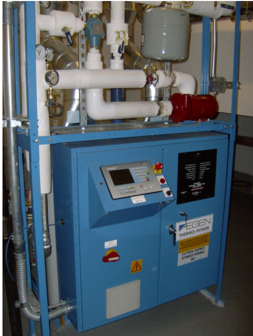
Figure 1. Aegis Energy Services AGEN-75 Engine Generator (1 of 2 typ)
