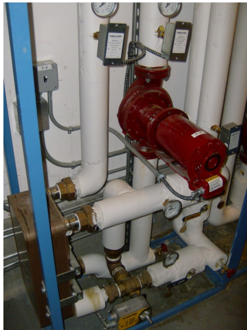
Building Heating Loop Pump P-4 and HX
