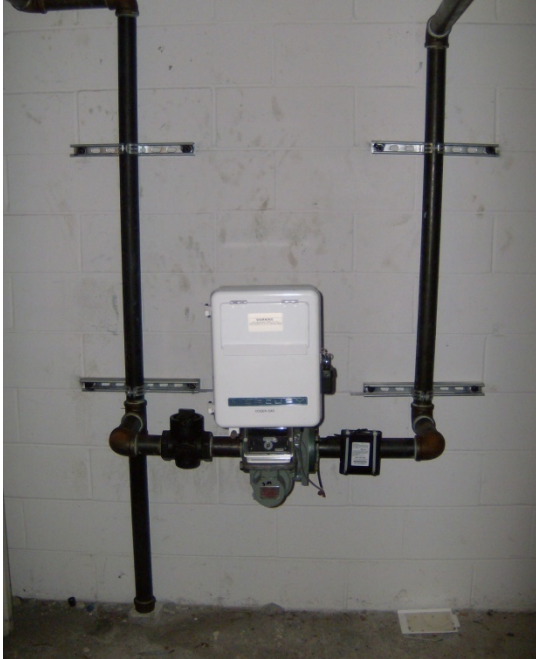
Figure 11. Utility Gas Meter In Basement Metering Room
