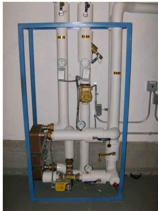
DHW High Zone Pump (P-6) and HX
