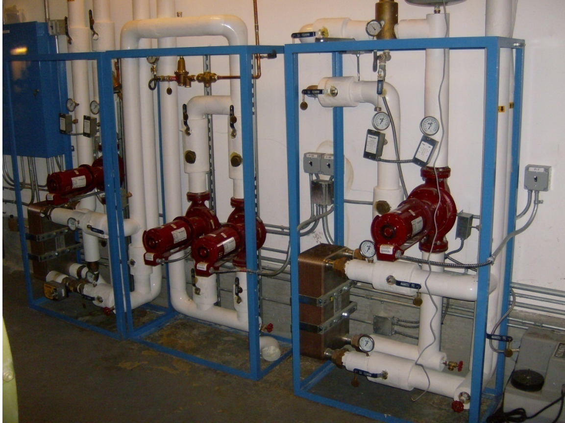
Figure 2. CHP Skid Heat Recovery Piping, Circulation Pumps, and HX
