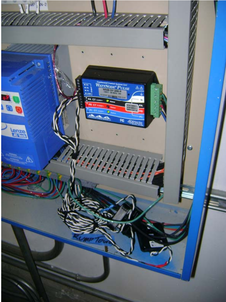
Figure B-4. Parasitic Power Watt-Node Power Transducer In 208 VAC panel
