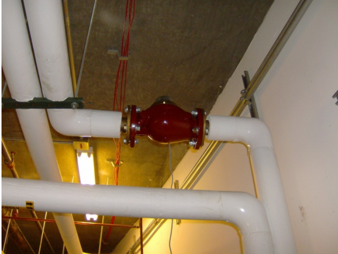
Figure 10. Heat Recovery Loop Flowmeter
