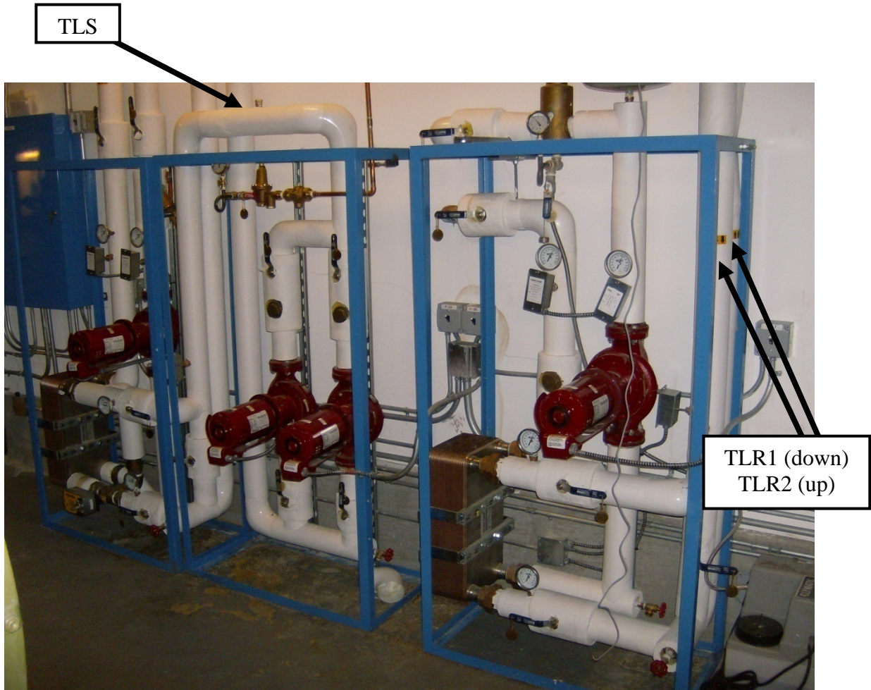
Figure 9. Location of Temperature Sensors on CHP Piping
