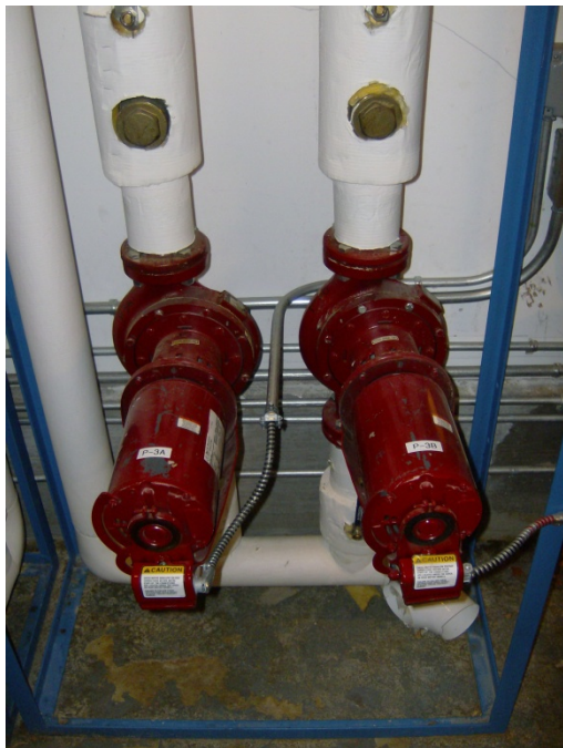
Primary Loop Pumps P-3a, P-3b
