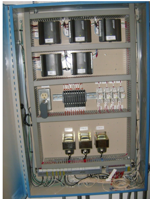
Aegis Communication Panel with 110 VAC Outlet
