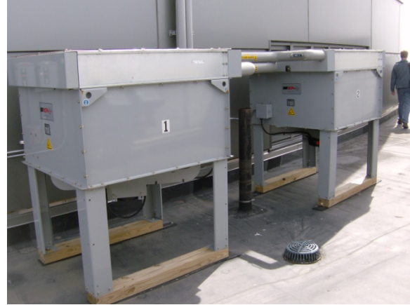
Dump Radiator Dry-Coolers
