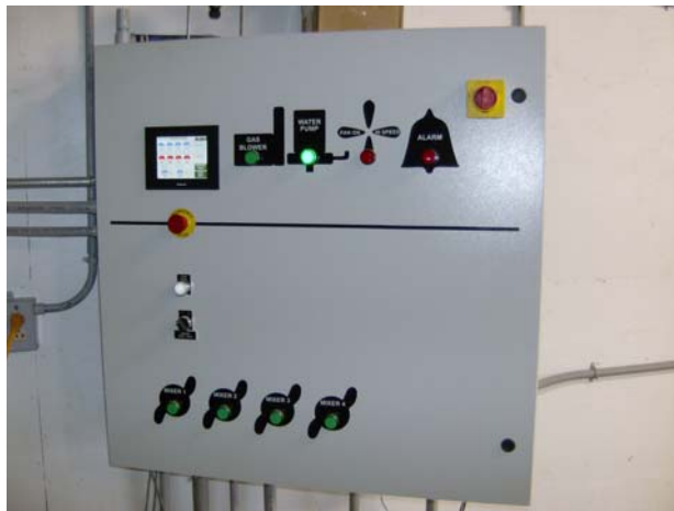
Digester control and status panel
