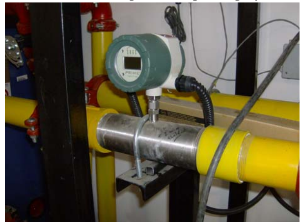
Sage Flowmeter – Biogas to engine
