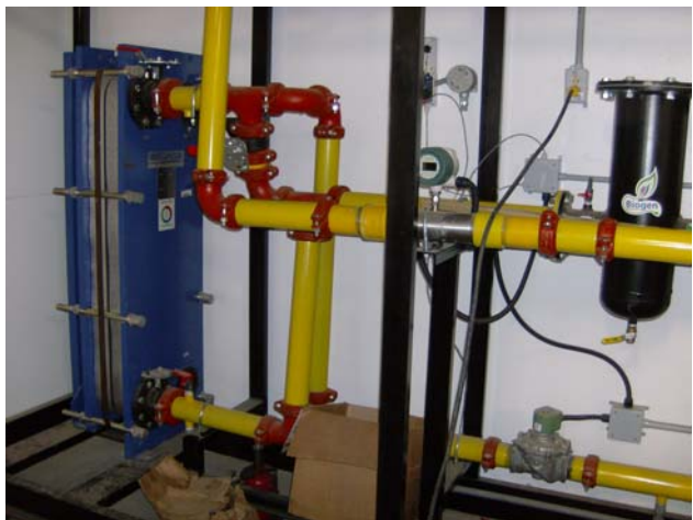
Biogas cooler and engine flow meter
