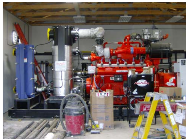
Genset – Guascor MGG-712 and heat recovery / hot water heat exchanger (left side, blue)
