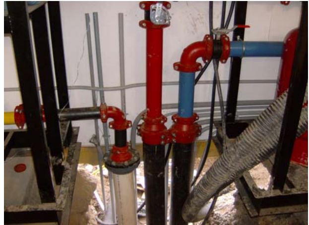
Piping – biogas to engine, hot water to digester, cold water from digester, temporary boiler exhaust (left to right)
