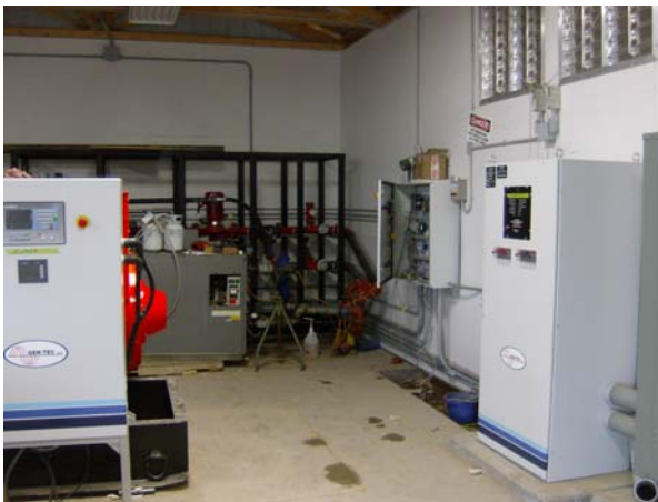
CDH panel will be on right wall between two existing panels.
