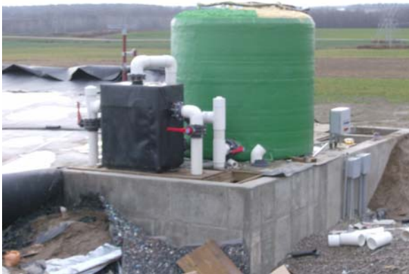
H 2 S Scrubber
