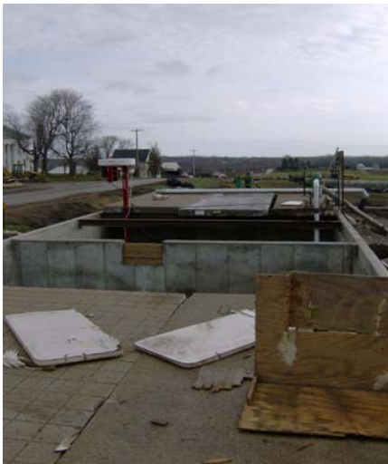
Cement storage tanks – 4x
