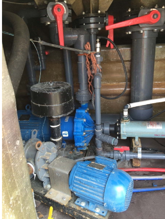
Air Blower & Recirculation Pump
