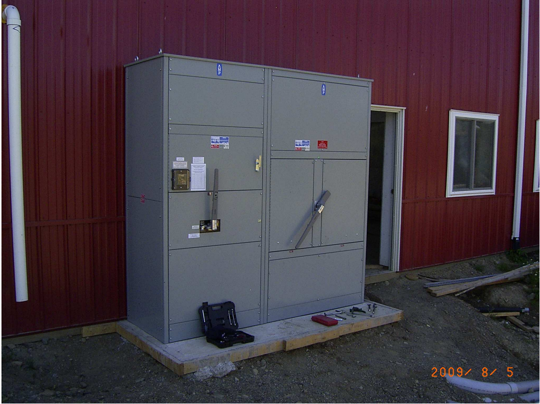
Breaker/Transfer Switch Gear Box
