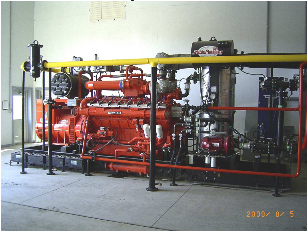
Biogas Engine Generator
