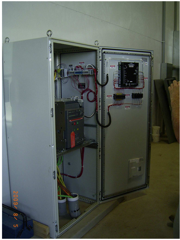
1,200 amp Breaker Box for Gen-Tec
