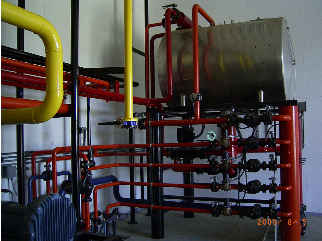
Red and blue heat exchange piping, water tank
