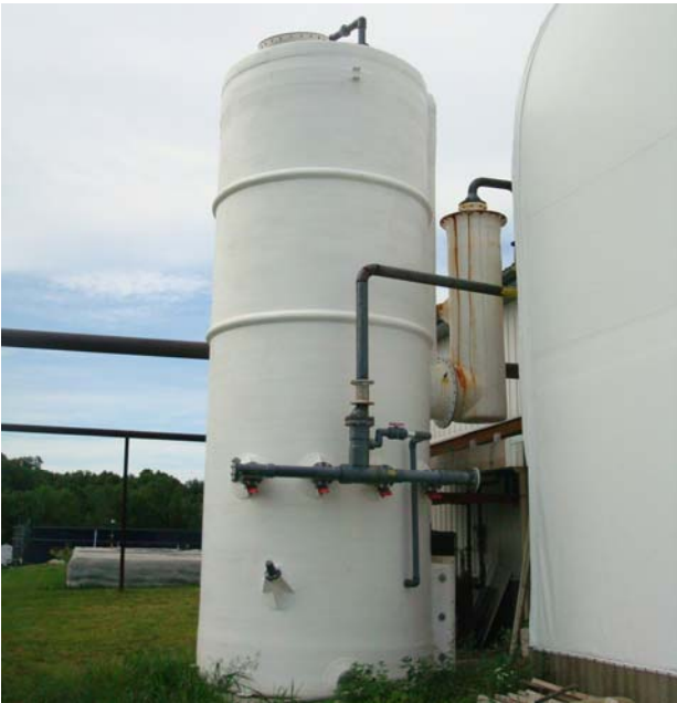
Energy Cube biological scrubber tower, located behind existing engine building.
