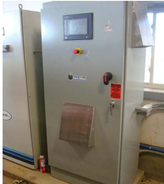
Scrubber control panel, located in existing engine building.
