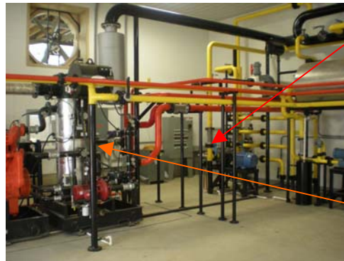
Heat Recovery and H2S Removal Equipment
