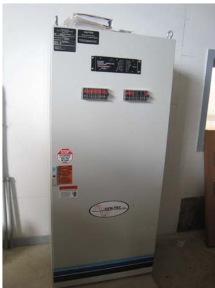
800 Amp Breaker for Engine Generator
