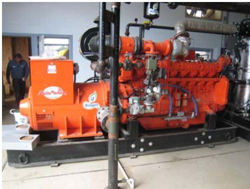
Guascor SFGLD 240 Engine-Generator
