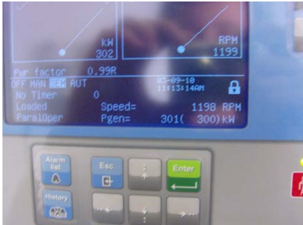
WG1 - Engine Control Panel
