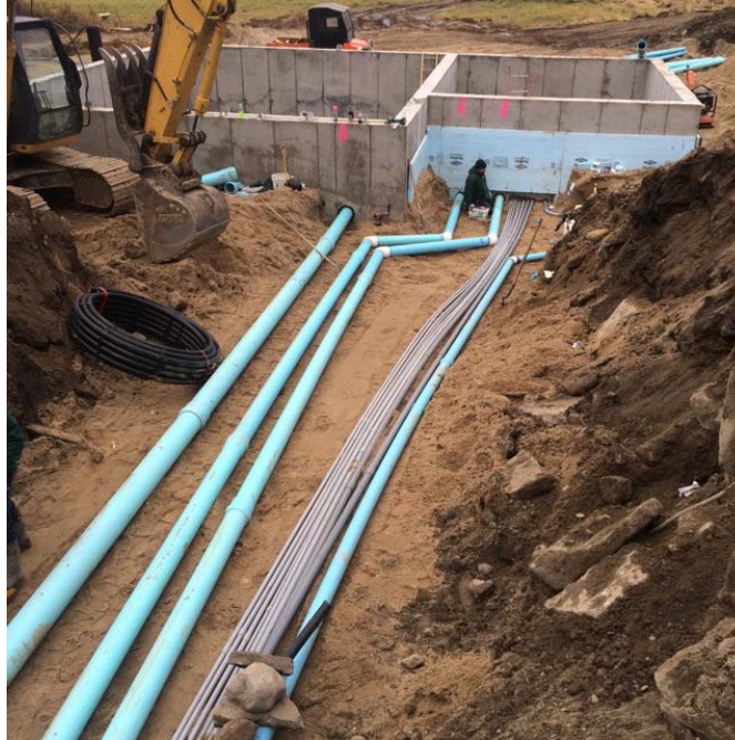
Figure 2: Manure Piping From Manure Pit
