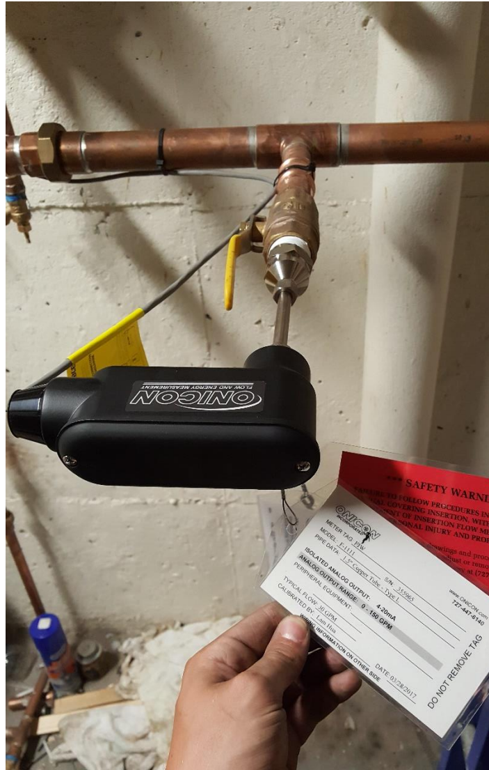
Onicon Flow Meter for Jacket Water Loop
