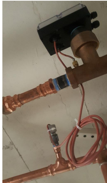
Badger BTU Meter for Exhaust Gas HW Loop
