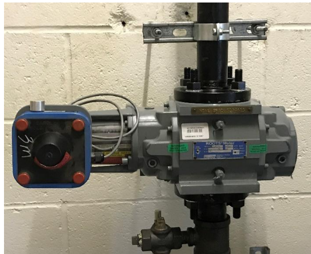
GE Roots Meter with 100CF/pulse pulse output (FG)
