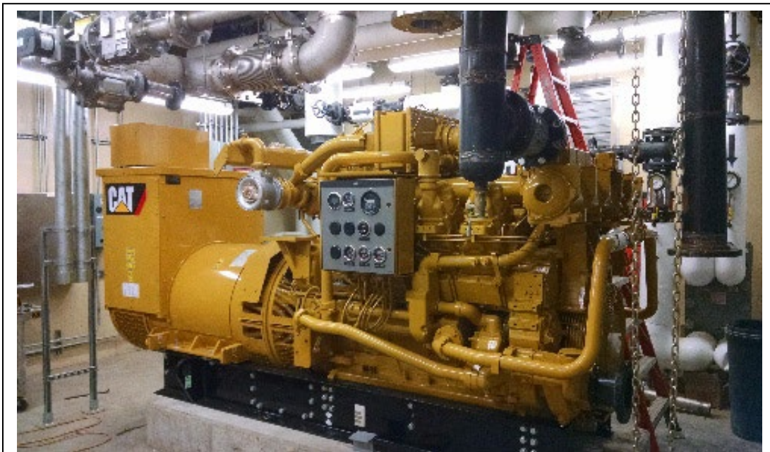
Figure 1: Caterpillar 375 kW Engine/Generator
