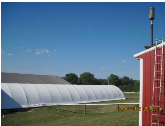
Digester and Flare
