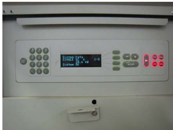
Micro-Turbine Control Panel
