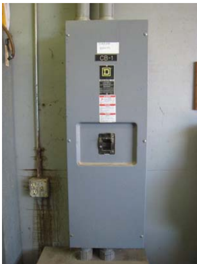
CB-1 400 A for digester and power generation
