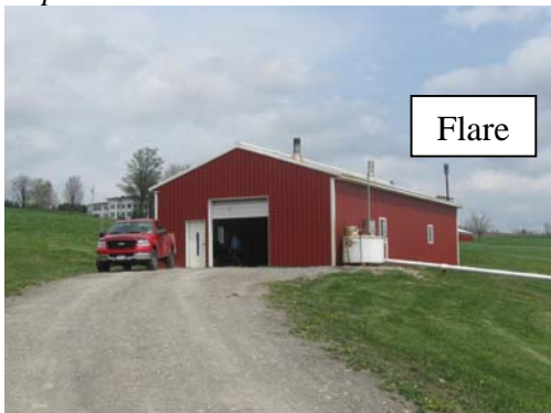
Pole Barn and Biogas Flare
