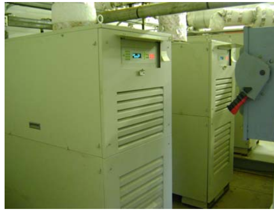
Capstone 30kW natural gas micro-turbines
