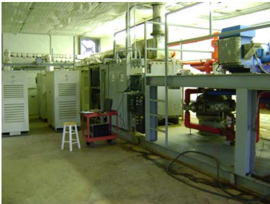
Digester House – Turbines (left), power meters (center), hot water loop equipment (right)
