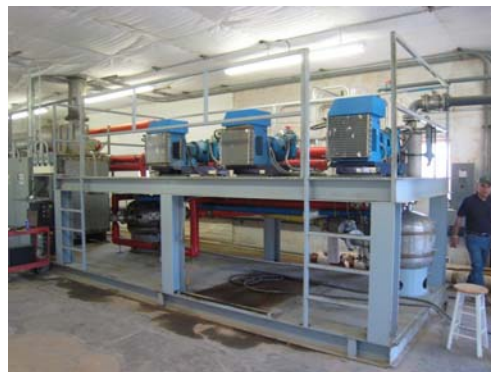
Biogas Conditioning Skid
