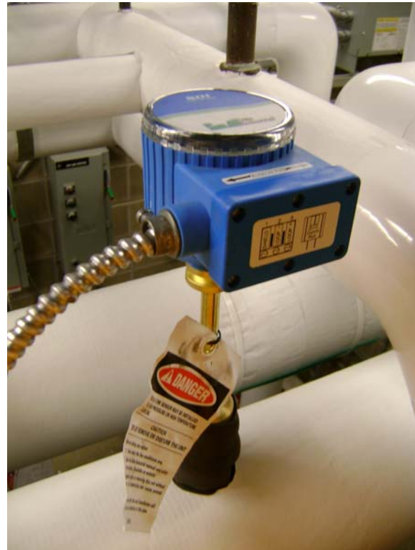
Chilled Water Flow Meter On Return Leg
