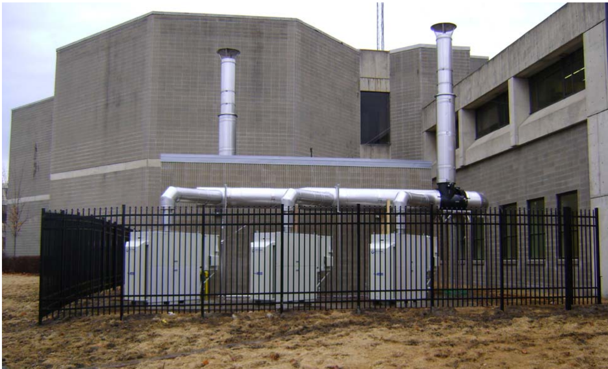
Figure 1. Microturbines and Chiller Building
