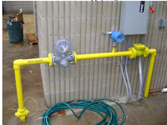
Gas Meter Installed on Gas Main Service to Microturbines For Combined Gas Consumption
