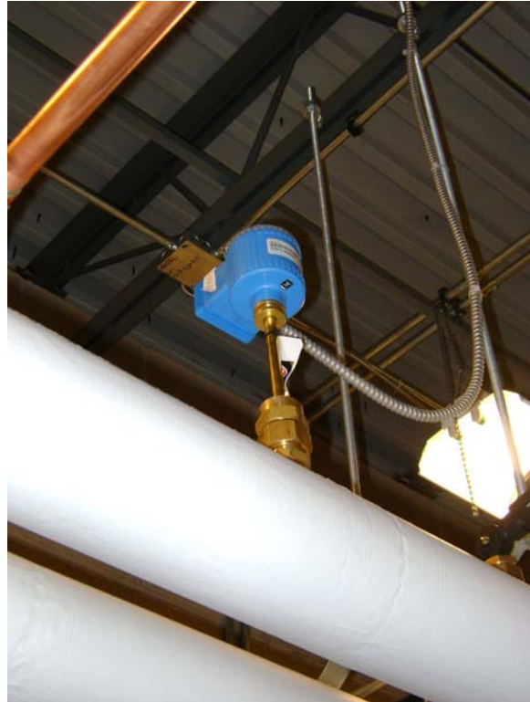
Hot Water Flow Meter on Supply Leg
