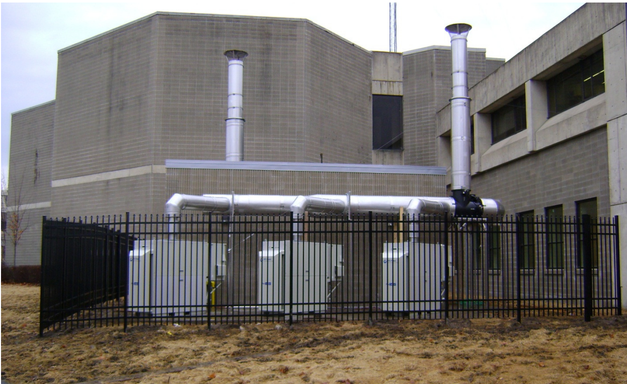
FIGURE 4 MICROTURBINES AND CHILLER BUILDING
