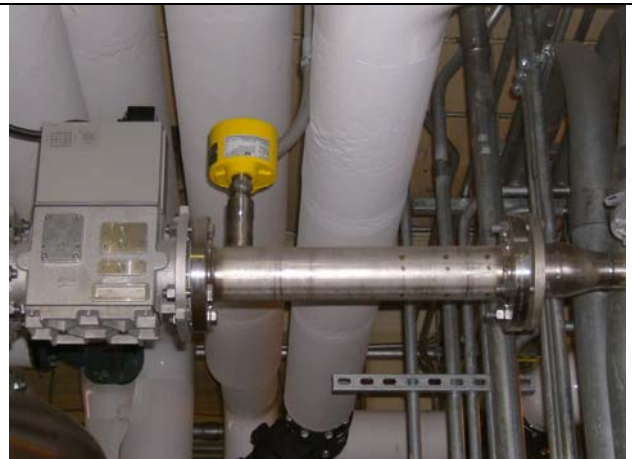
Biogas flowmeter - one (1) per engine
