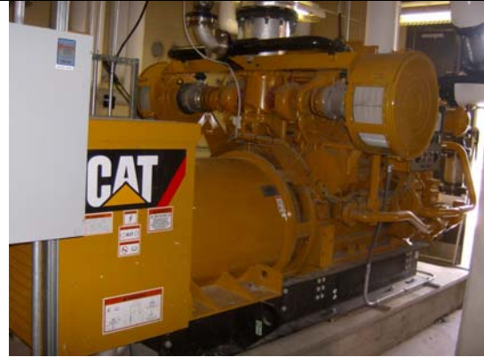
Caterpillar engine / generator. Both are identical.
