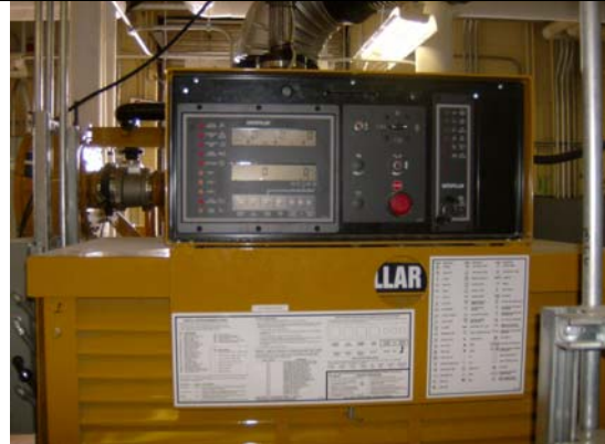
Generator display / power quality
