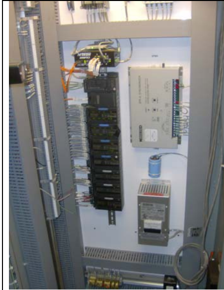
Inside PLC / control system panel. Pulse outputs wired on left - TM4, inputs 17-20
