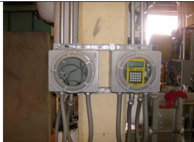
Biogas flow meter displays - one currently installed.
