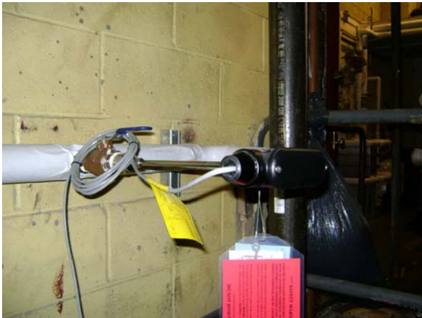
FB – Behind boilers just to the left of TBR sensor
