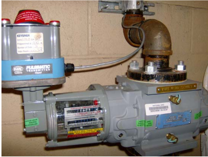
Gas Meter with new Head Installed
