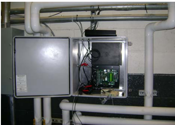
Obvius Datalogger Box – Mounted on the right wall when looking in generator room from outside.
