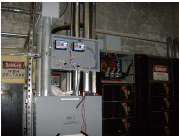
WE1 and WE2 – in front of boilers, in small box mounted above head height.
