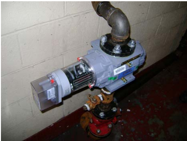
FG – in narrow side room, off of large boiler room, against right wall
