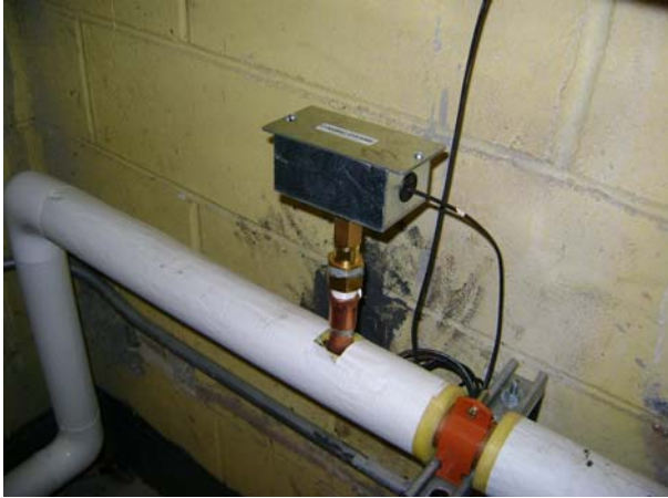
THR2 – Behind boilers, bottom left corner of wall.
