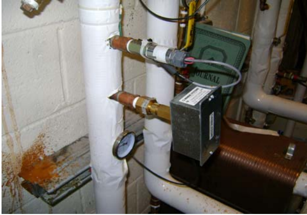
THS – on HX wall, left most and lower of the THR1 temp sensor.
