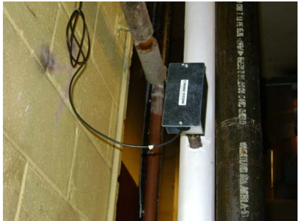
TBS – Behind boilers, right side of wall, above TBR
