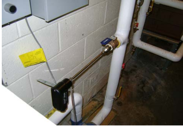
FW – on HX wall below expansion board box (grey in upper left corner of pic)
