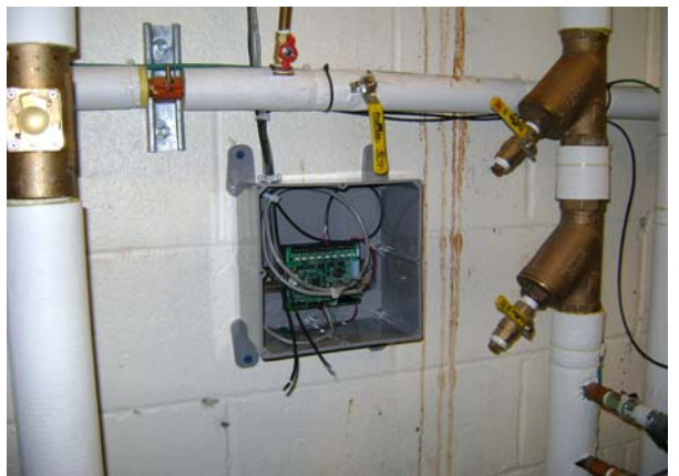
Obvius Expansion Board Box – Mounted on HX wall.
