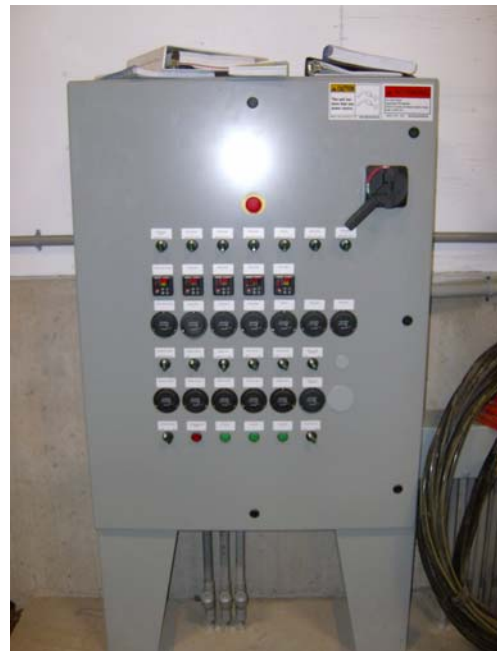
Digester Temperature Control Panel
