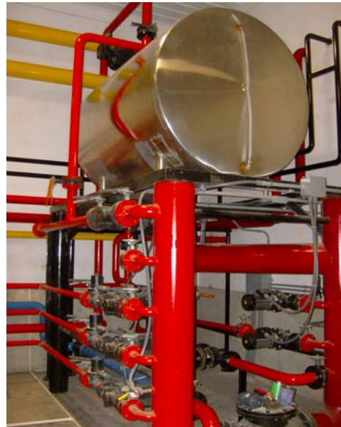
Hot water storage tank and piping
