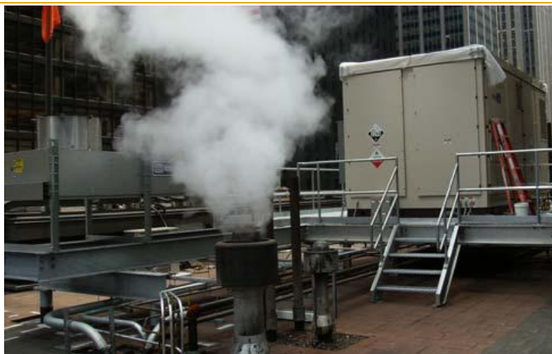
FIGURE 6 INSTALLED FUEL CELL AND DRY COOLER ON LEFT
