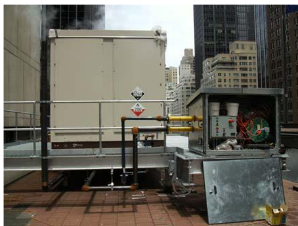
FIGURE 3 INSTALLED FUEL CELL AND GAS BOOSTER
