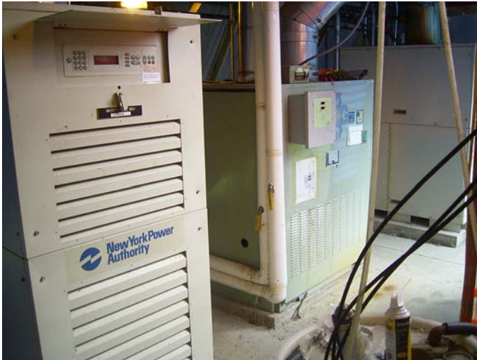
MT #1, Air to Liquid Heat Exchanger, MT #2
