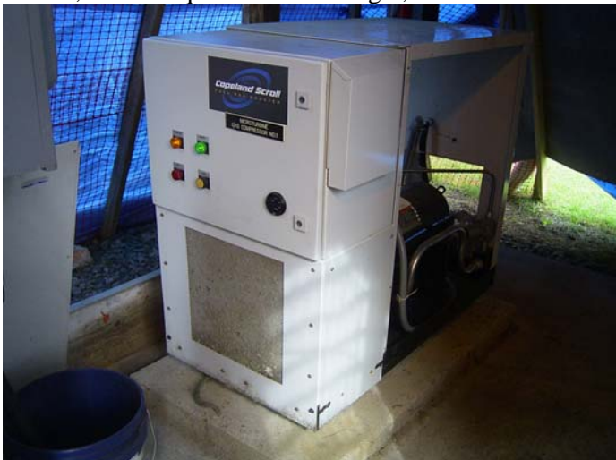
MT #1 Gas Compressor
