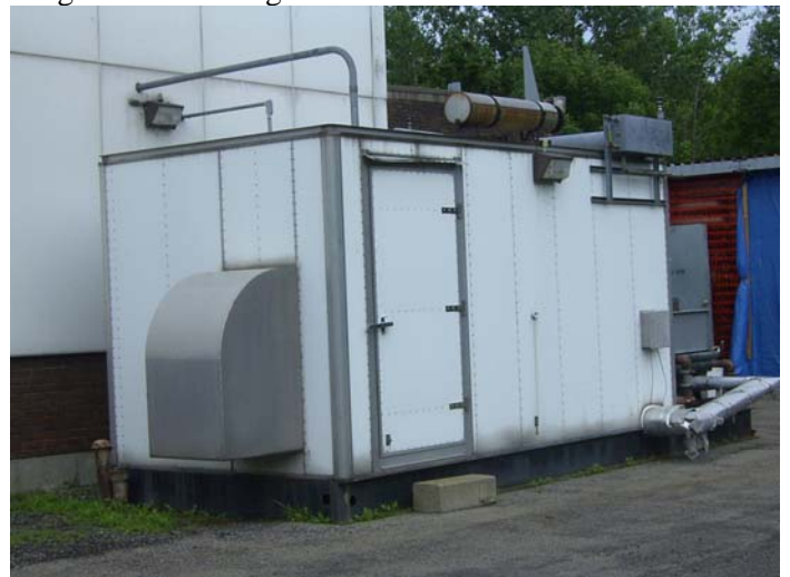
Backup 100kW Generator
