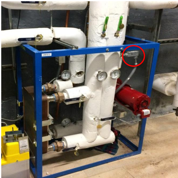
Veris 10K Type II Thermistor (THW3) on Dump Radiator skid after HX2 located in boiler room.
