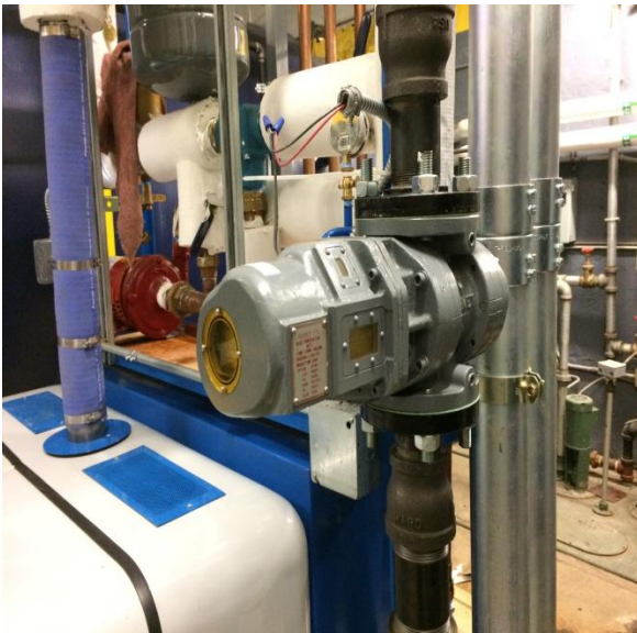
Romet RM2000 gas meter (FG) located on cogen unit skid.
