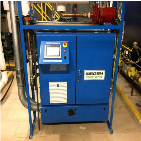
Aegen PowerVerter 100 kW cogen unit located in the boiler room.
