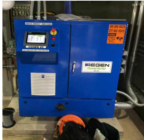
Aegen PowerVerter 100 kW cogen unit #2 located in the boiler room.
