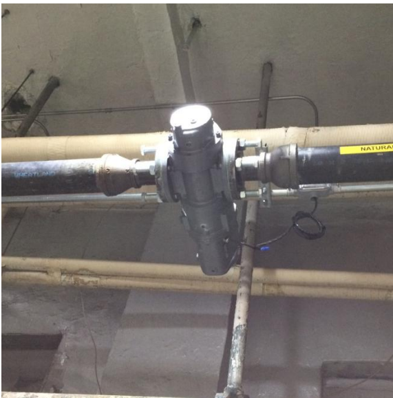
Romet RM3000 gas meter (FG) for both cogen units 1 & 2
