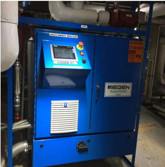
Aegen PowerVerter 100 kW cogen unit #1 located in the boiler room.
