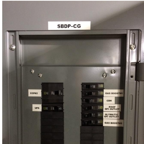
Parasitic power (WP) measured from sub-basement distribution panel CG located through double doors on the left side of the electrical room adjacent to the boiler room.
