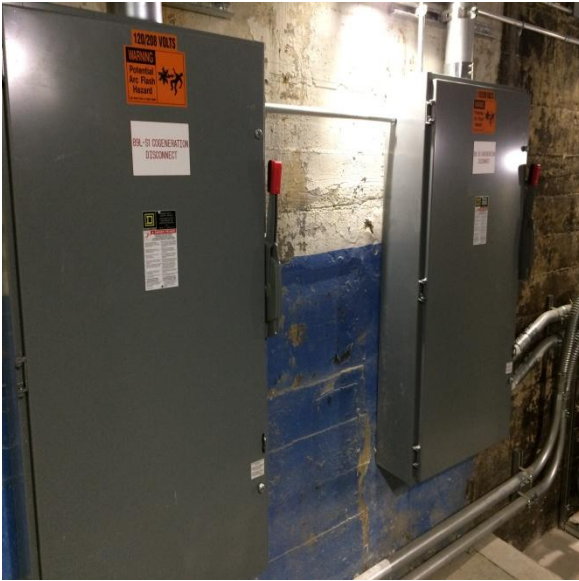
Gross generator power meter (WT1, WT2) located in cogen disconnects through the double doors on the left side of the electrical room adjacent to the boiler room.
