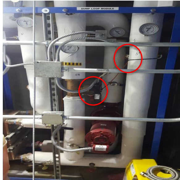
Dump Radiator Skid - Located in Boiler Room Left - BTU meter and temp. sensor after DHW HX1 (THW2) Right - BTU temp. sensor after dump radiator HX2 (FHW ,THW3)
