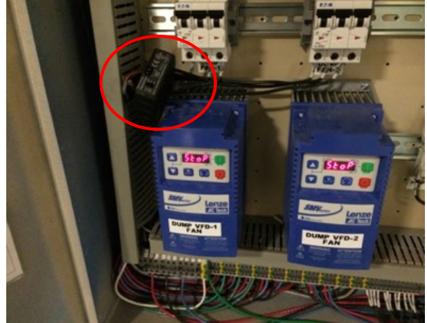
Veris H921 current sensor (IVFD), located in Aegis control panel.
