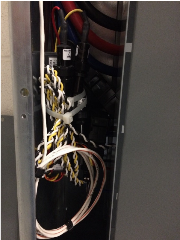
Parasitic power meter (WP) located in SBDP-A subpanel in the electrical room.
