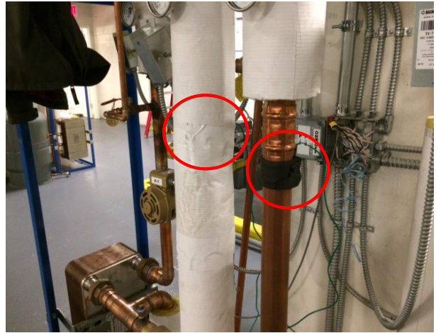
Two Veris 10k Type 2 Surface Thermistor (THW2 & THW3), located in the boiler room on DHW module across HX4 and HX5.
