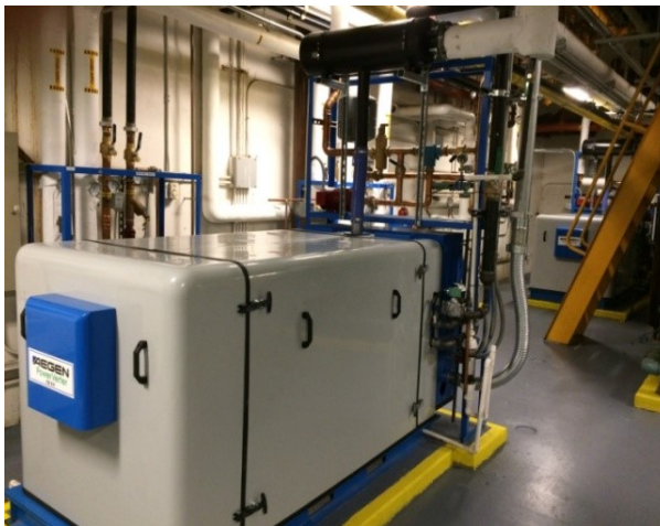
One of Two Aegen PowerVerter 100 kW cogen units located in the boiler room.
