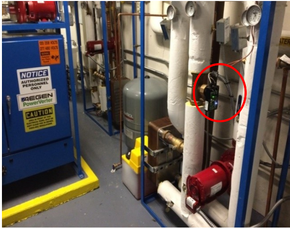
Badger 380 BTU meter on the dump radiator module (THW4, THW5, FHW).
