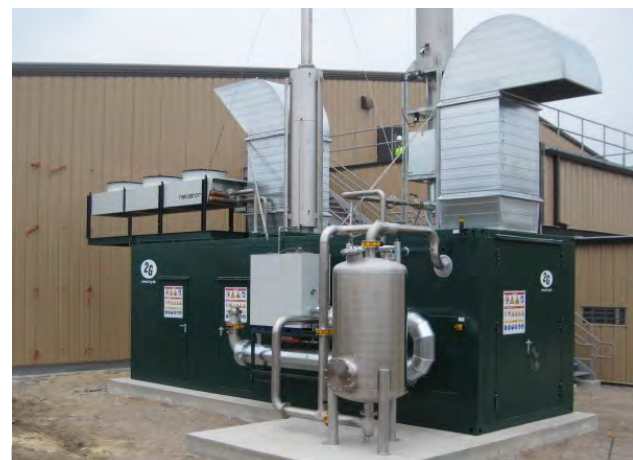
Municipal Dry Anaerobic Digester Biogas CHP Power Generation Plant with “Plug & Play” Container Module, including Gas Conditioning & Treatment System.
