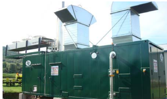
Enclosure housing engine, generator, hot water heat recovery, gas analyzer, and power and gas metering equipment.
