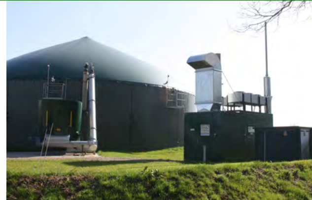
Anaerobic Farm Digester Biogas CHP Power Generation Plant with “Plug & Play” Container Module.
