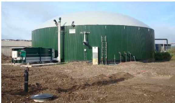
Newly installed fully mixed, soft cover, heated, PlanET digester; 82 ft ø, 26ft tall.
