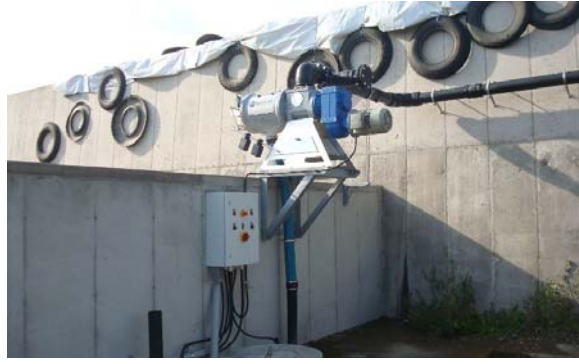
Digester effluent solids / liquids separator.
