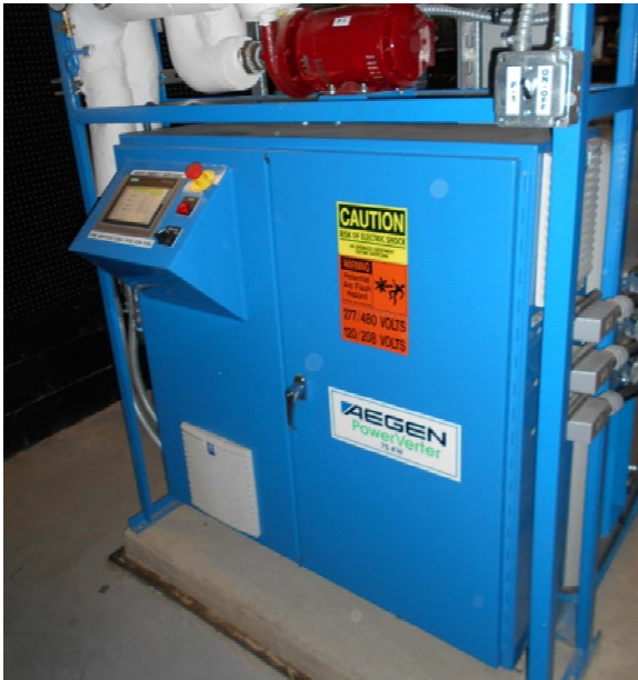
Aegen Powerverter cogen unit located adjacent to sub-basement boiler room.
