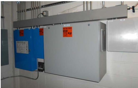
Aegis control panel (left), cogen UPS (center), and CDH panel (right).
