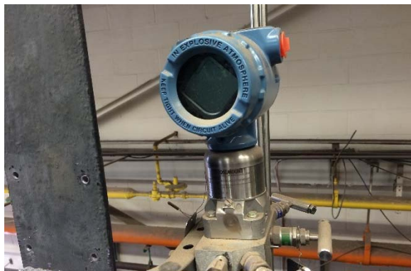
Steam Flowmeter Display (FS)
