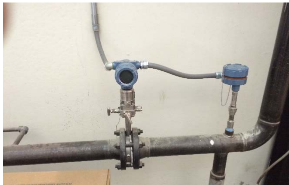
Duct Burner Gas Meter (FGDB)
