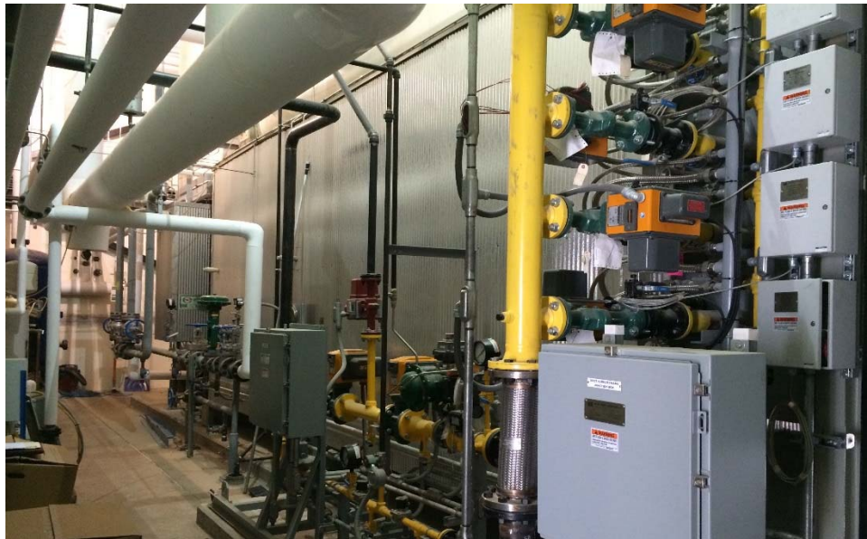
Heat Recovery Steam Generator (HRSG)
