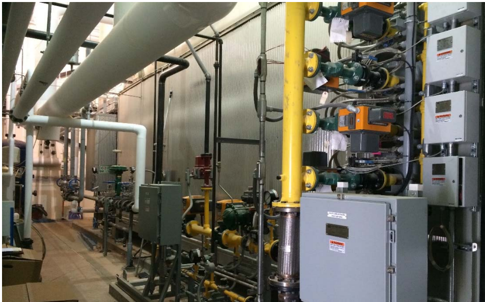
Heat Recovery Steam Generator (HRSG)
