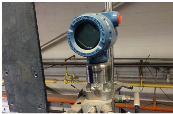
Steam Flowmeter Display (FS)
