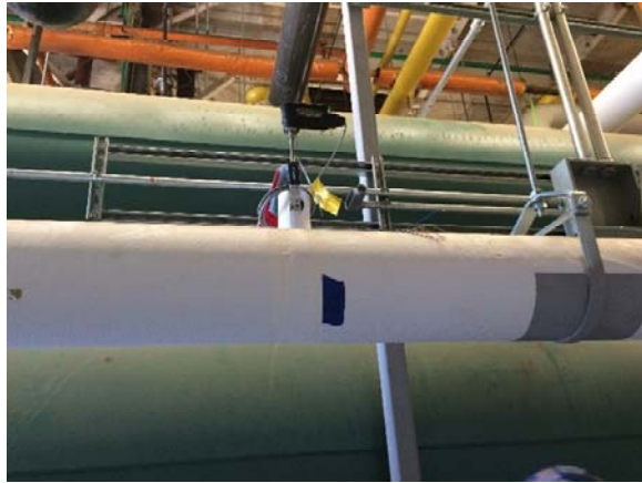
Chilled Water Flow Meter
