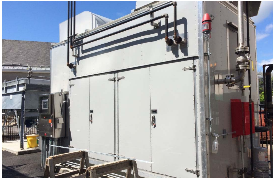
Gas Compressor Enclosure (next to gas turbine skid)
