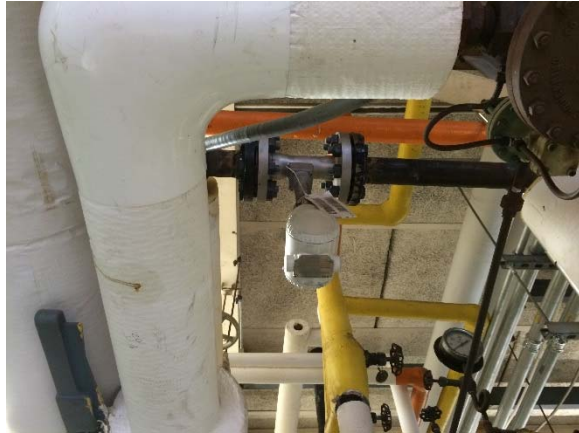
High Pressure Deaerator Steam Flow Meter (FSDAHP)
