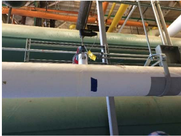
Chilled Water Flow Meter
