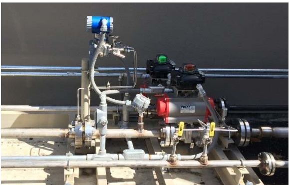
Turbine Gas Meter (FGT)
