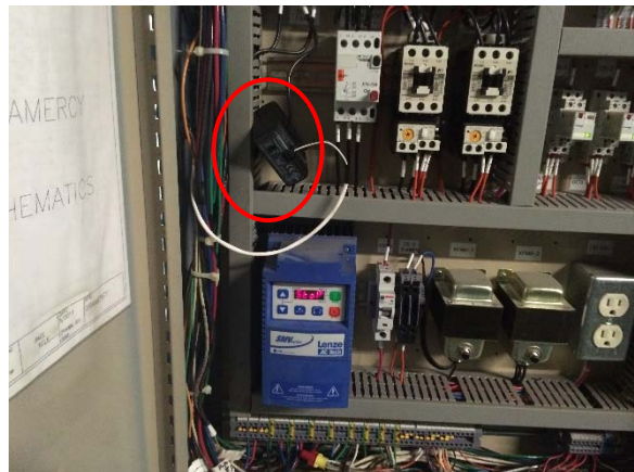
Dump radiator fan current sensor.
