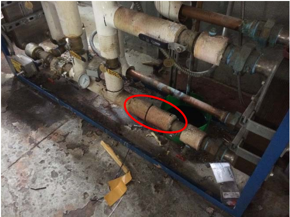
Location of Veris Thermistor between HX1 and dump radiator HX on new cogen loop.
