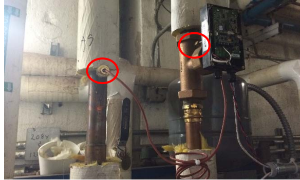
New cogen Badger 380 BTU meter, measuring total heat recovery (temp sensors circled).
