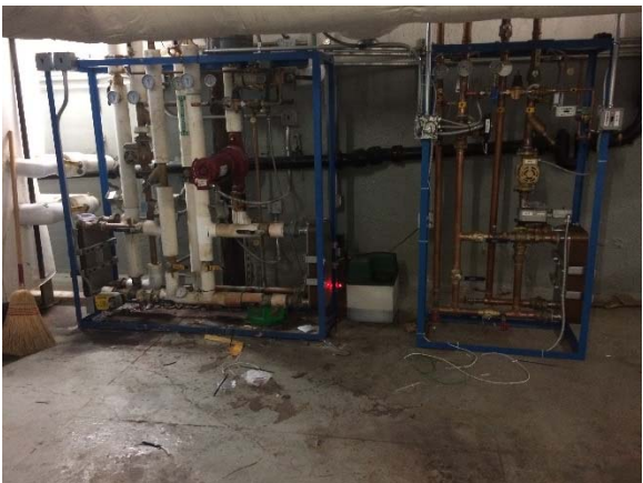
New cogen unit HX skid (left) and existing cogen unit HX skid (right).
