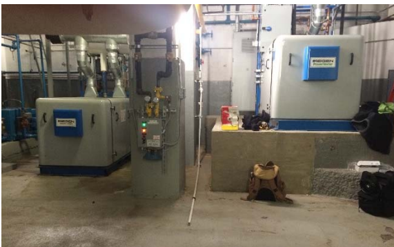
Aegen TP75-LE cogen units located in basement mechanical room; existing (left) and new (right).
