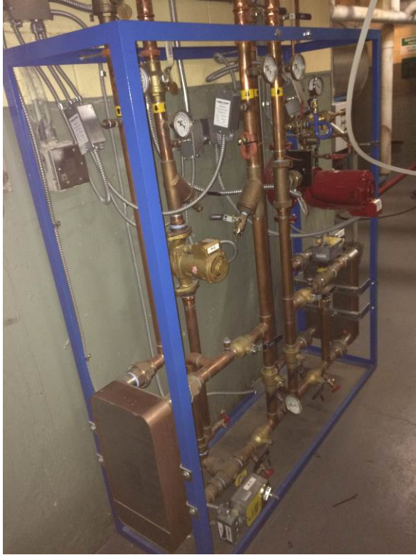
Heat recovery HXs (2)
