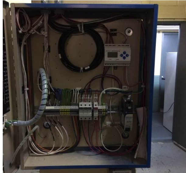
Veris E50 power meter (WB) in Beckwith panel located in cogen room.
