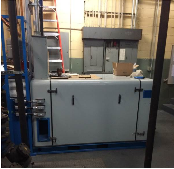
One (1) Aegen Powerverter (PV-75) cogen unit located in cogen room in basement
