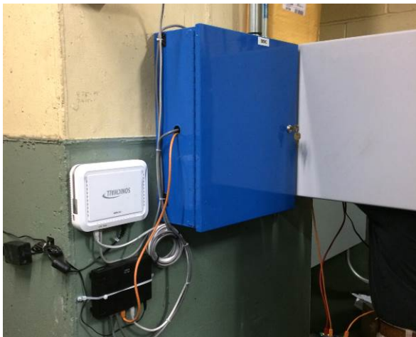
CDH panel containing Obvius data logger (right) and Aegis CCP1 and network equipment (left).
