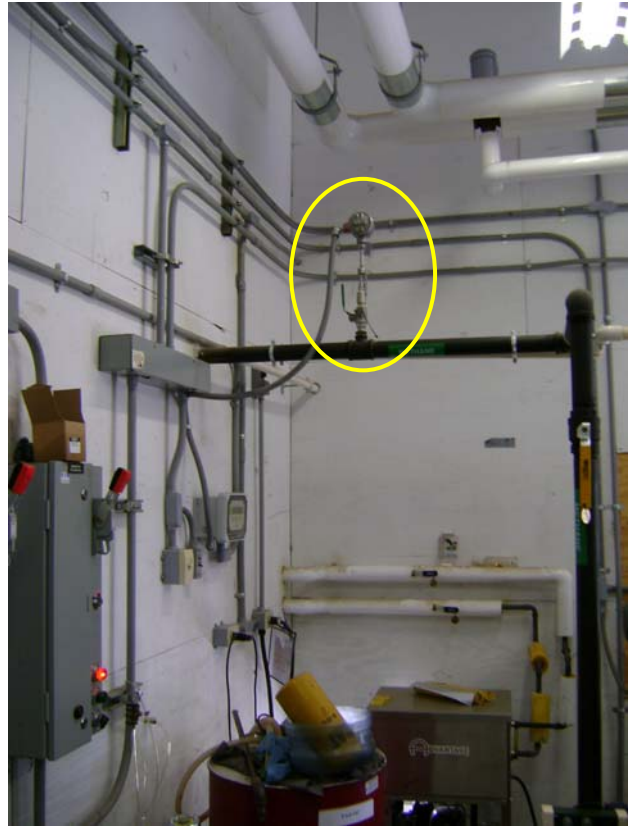
Sage Gas Flow Meter - #2 (flow to engine)
