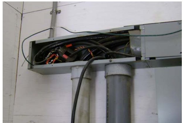
Veris Power Meters (measuring power use in back dairy barn, EP-2 on the Display; EP-4 at Breaker)
