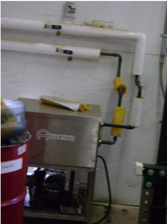
Biogas Conditioning - Chiller
