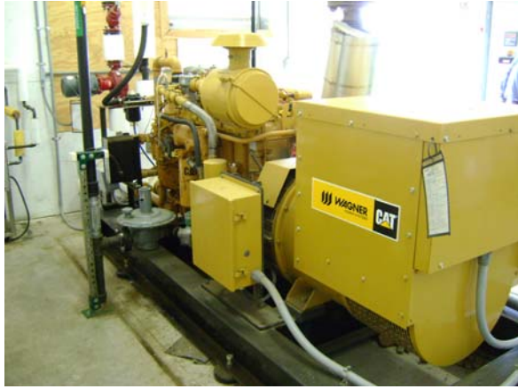
Caterpillar engine and generator
