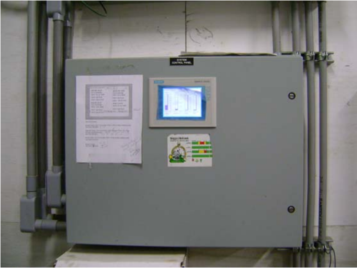
Electric control panel, Siemens PLC, and Touch Screen
