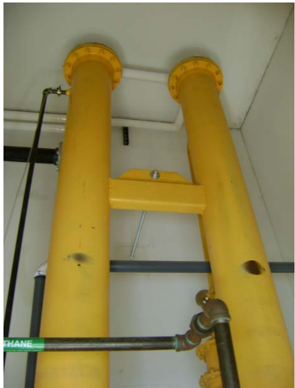
Biogas Conditioning – shell and tube heat exchanger
