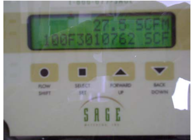
Sage Display (FG2) – Biogas flow to engine
