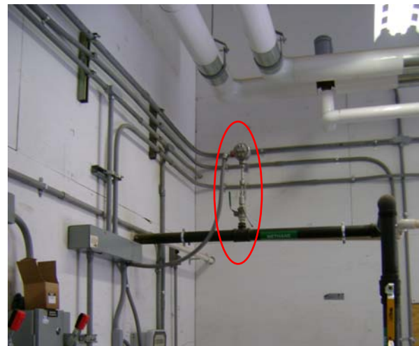
Sage Flow Meter (FG2) – biogas flow to engine
