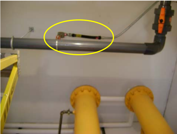
Sage Gas Flow Meter - #1 (total gas flow)
