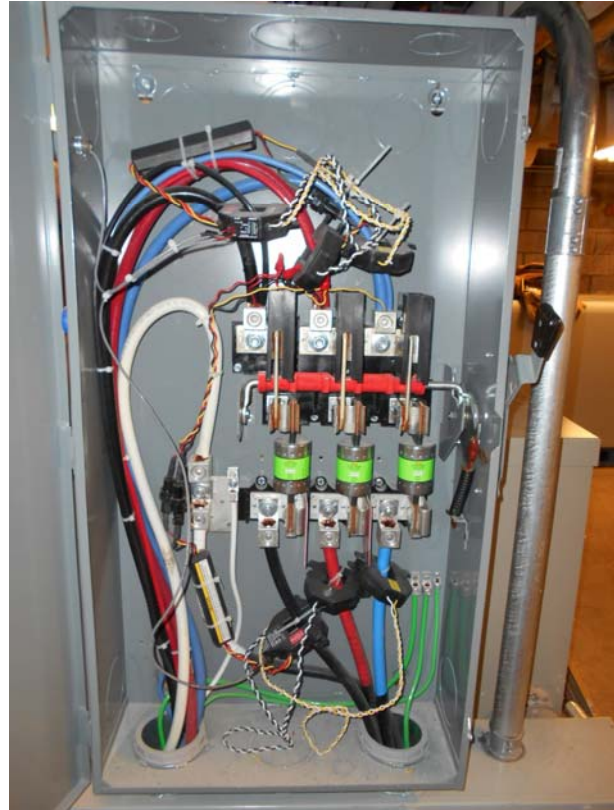
Veris H8035-300 power meter (WT) located in generator disconnect in cogen room (BOTTOM).
