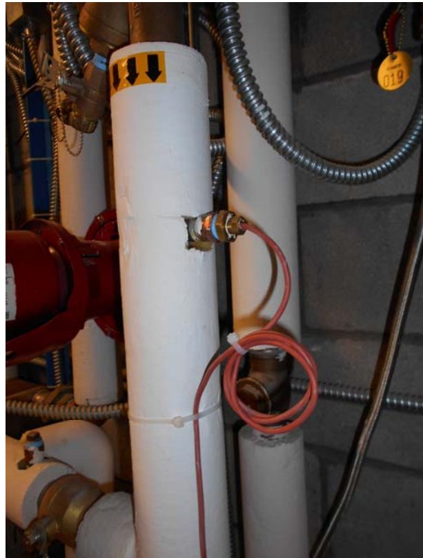
THW1 CHP Supply (BTU is on QU)
