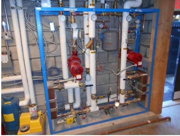
Single heat recovery HX and dump HX skid
