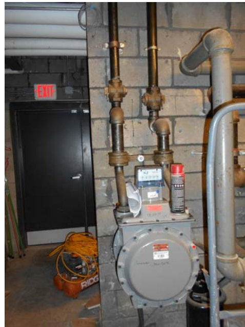
Cogen utility gas meter (no pulser) and wire run
