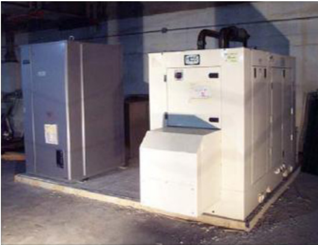
FIGURE 5 GENERATOR (RIGHT) AND ABSORPTION CHILLER (LEFT)
