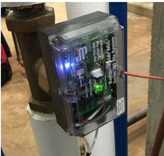
Badger 380 BTU meter (THW1, THW3, FHW).
