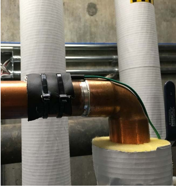
Veris 10k Type 2 Thermistor (THW2), located in mechanical room.
