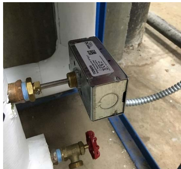
Mamac 10k Type 2 Thermistor (THW4), located in mechanical room.
