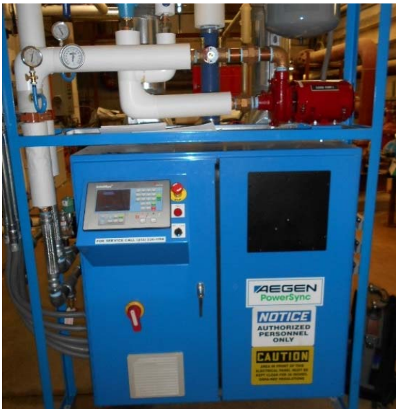
Aegen TP75-LE cogen unit located in basement mechanical room.
