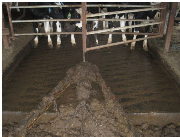
Existing Manure Scrape System.
