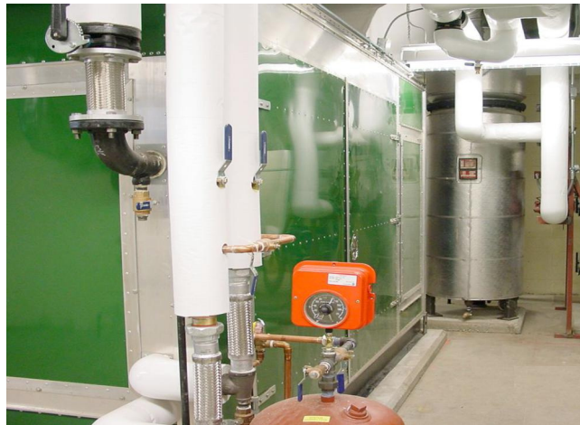
FIGURE 5 EXHAUST HEAT RECOVERY UNIT AT REAR OF ENGINE
