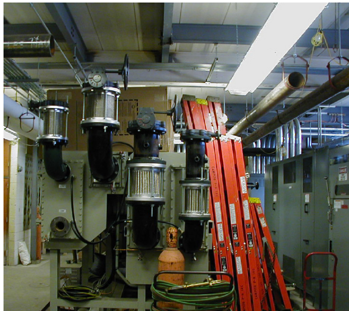
FIGURE 6 ABSORPTION CHILLER PROVIDES AIR CONDITIONING
