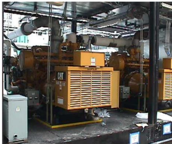
FIGURE 3 ENGINE MODULES INSTALLED SIDE-BY-SIDE ON ROOF
