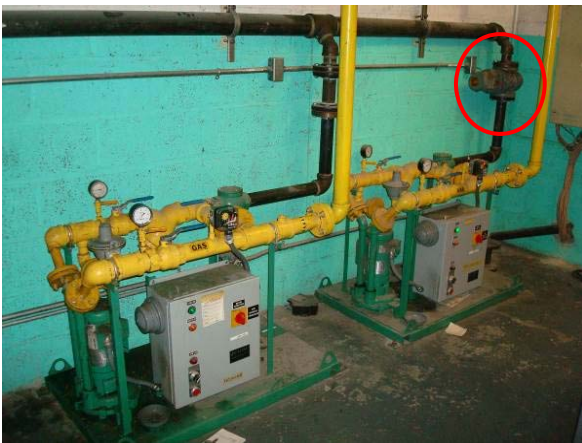
Gas boosters for both cogen units, and Romet RM2000 gas meter for one cogen unit, only FG1 wired / functioning.
