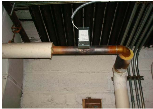
Mamac 10k Type 2 temperature sensor (THW2), installed by Aegis.
