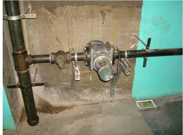
Roots rotary gas meter with pulse output. Meter measures total gas input to both cogen units (FGT).
