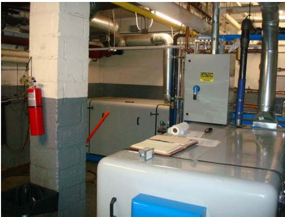
Aegen Powerverter 75 cogen units (2x) located in basement mechanical room.
