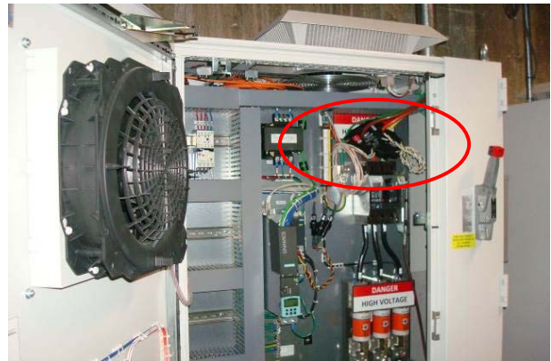
Veris H8035 power meter (WT1, WT2); located in each inverter.
