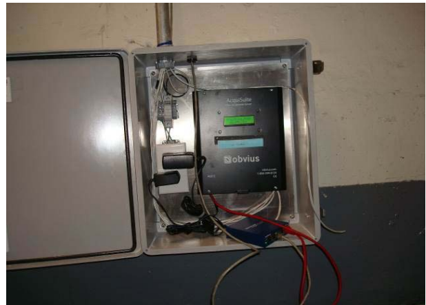
CDH panel containing data logger and CDH network switch.
