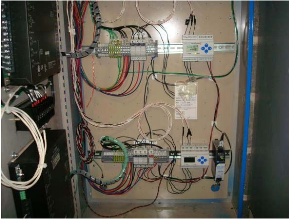
Veris E50 power meters for total facility power measurement (WB1, WB2), located in Aegis panel next to UPS.
