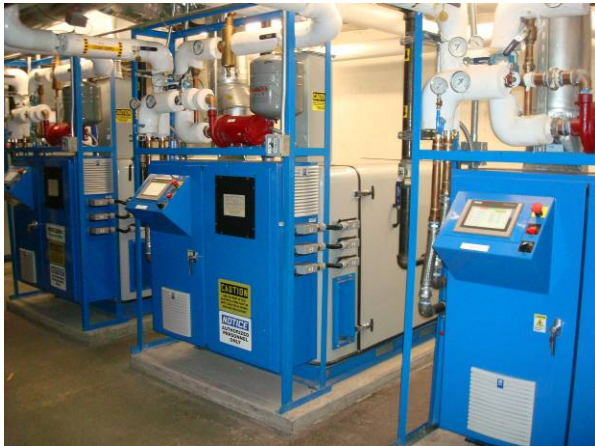
Three (3) Aegen Powerverter (PV-75) cogen units located in cogen room in sub-basement level parking garage.
