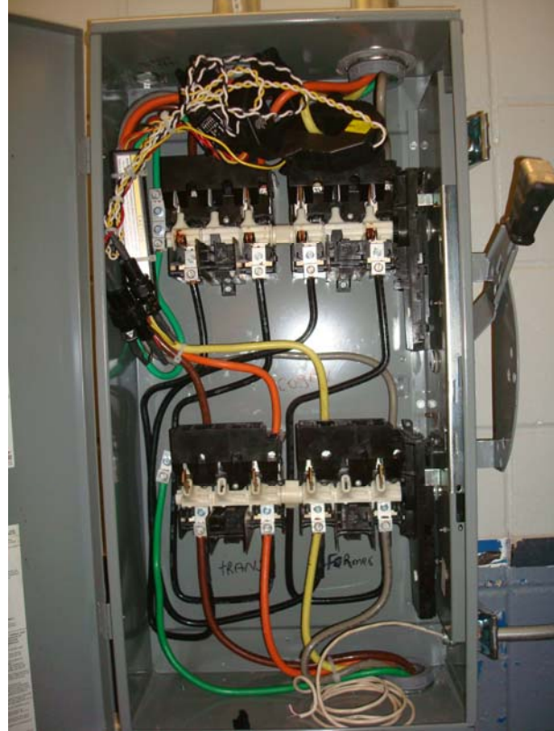
Veris H8035-100 power meter (WP) located in manual transfer switch in basement hallway.
