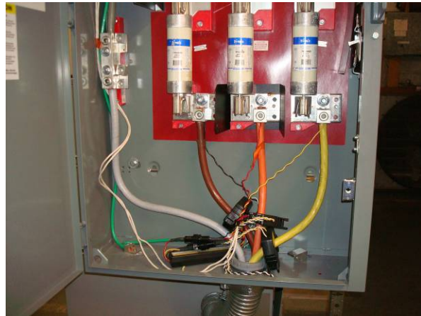
Veris H8035-300 power meter (WT23) located in generator #2 & #3 disconnect in cogen room.
