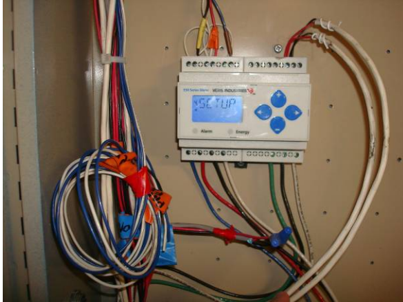
Veris E50C2A power meter, 1 of 2 typ. (WB1, WB2) located in basement electrical motor room (WB1) and 8th floor mechanical room (WB2).
