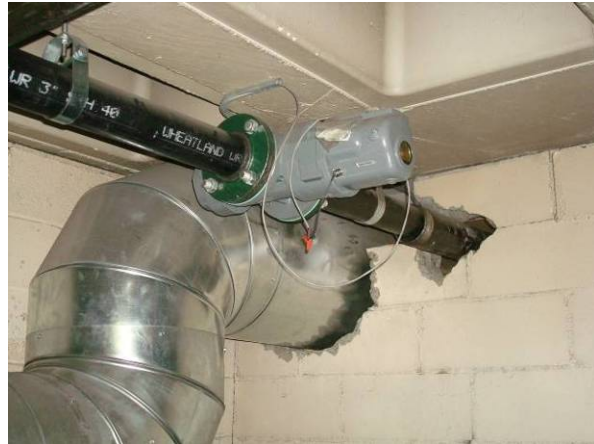
Romet RM5000 rotary gas meter (FG) with pulse output located in sub-basement parking garage outside cogen room.
