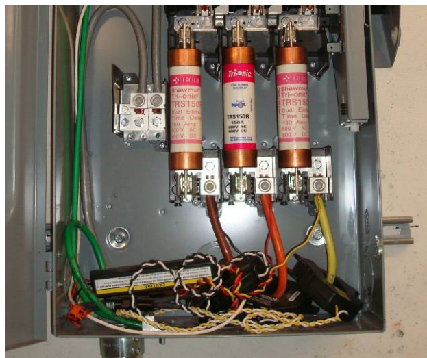
Veris H8035-300 power meter (WT3) located in generator #1 disconnect in cogen room.
