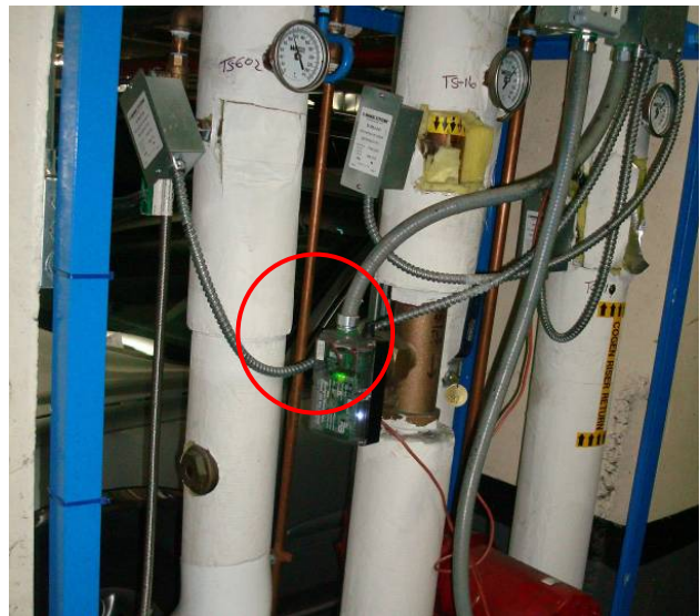
Badger 380 BTU meter (FHW, THW2, THW3) located in sub-basement parking garage outside cogen room.
