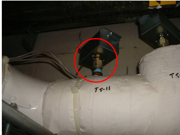
Recovered heat loop temperature sensor (THW1) located above HX's on load side piping in cogen room.
