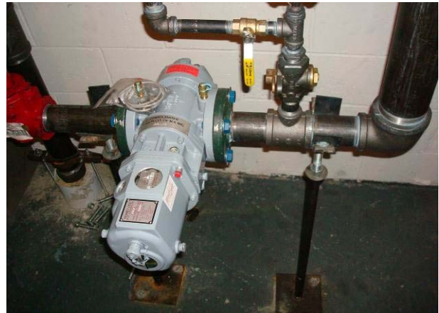
Romet RM2000 utility gas meter w/ pulse output (FG) – located in basement gas meter room.
