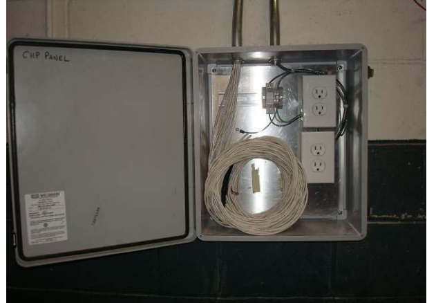
CDH panel, located in basement mechanical room.
