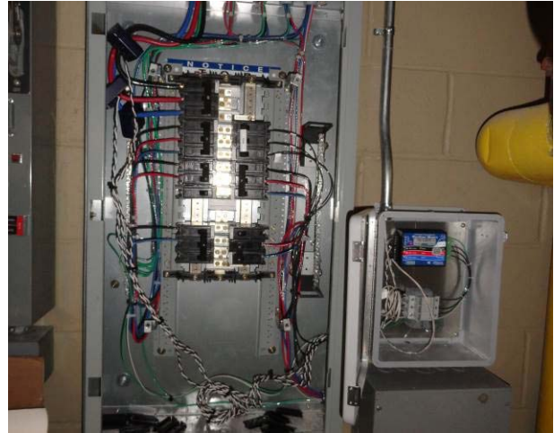
Parasitic load panel (left) and Wattnode WMB power meter (WP) – located in penthouse mechanical room.
