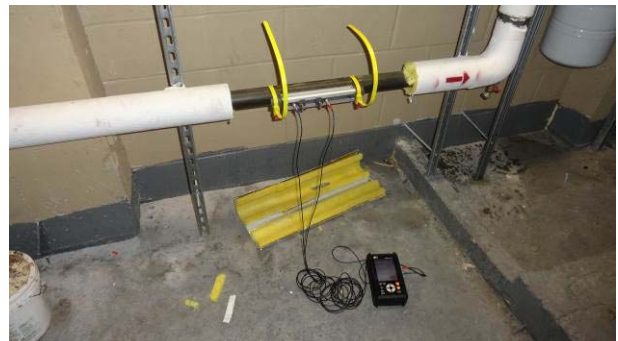
Portaflow ultrasonic flow verification location for dump loop flow (FHWD).
