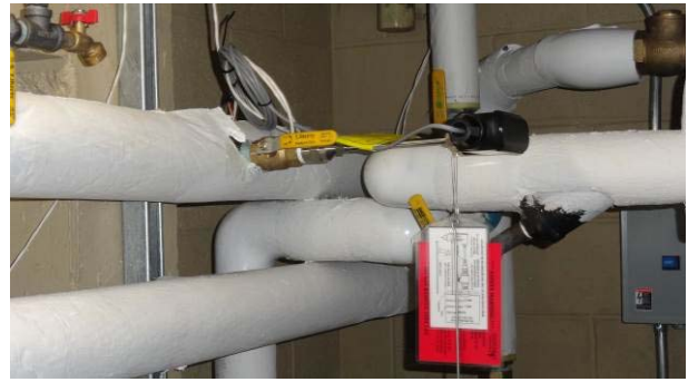
Dump radiator loop flow meter (FHWD) – in penthouse mechanical room.
