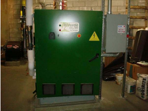
Tecogen InVerde 100 kW cogen unit located in basement mechanical room.
