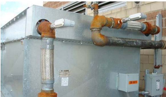
Dump loop supply and return temperature sensors (TDS, TDR) – located on penthouse roof.
