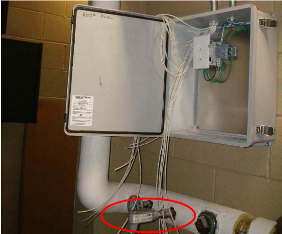
CDH panel for Obvius expansion board and cogen loop return temperature (THW9) – located in penthouse mechanical room.
