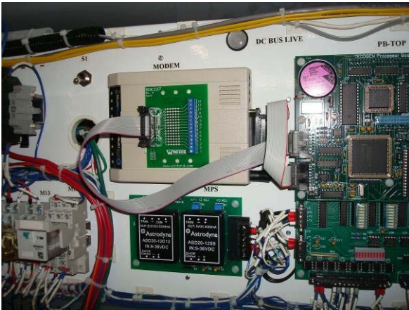
Modbus board installed in Tecogen InVerde 100 kW cogen unit electrical cabinet (WT) - located in basement mechanical room.
