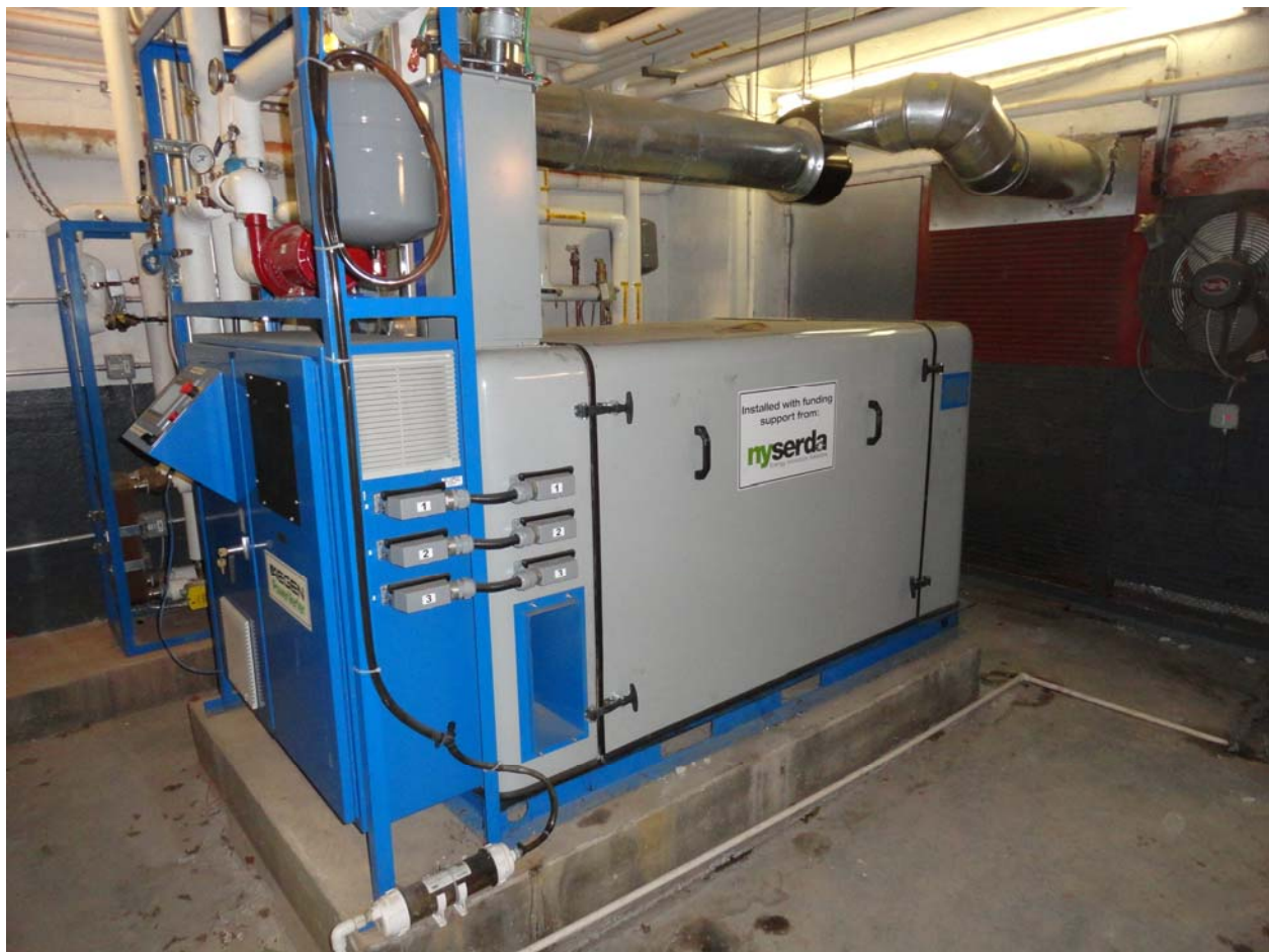
Figure 1. Birchwood Apartments – The Toledo Cogen Unit
