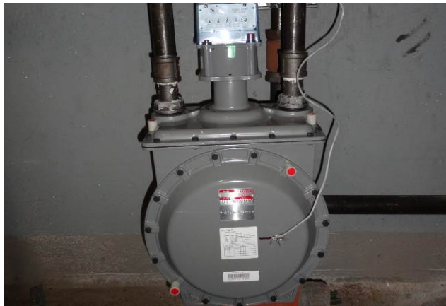
Utility gas meter, located in parking garage (FG)
