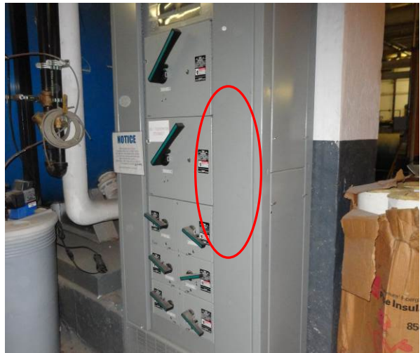
Location of cogen power meter (WG)
