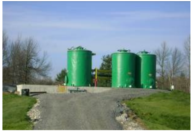
Installed biological scrubbers (2x) and iron sponge tank.
