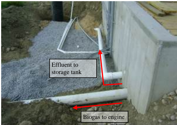
Buried effluent and biogas piping (from side of scrubber platform).
