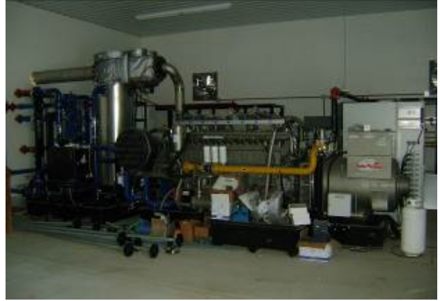
Installed engine and generator
