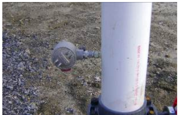
Flare gas flow meter.
