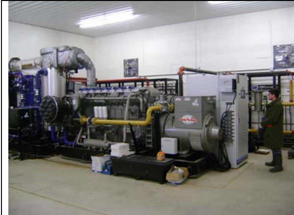
Guascor MGG-500 engine and Stamford HCM636J generator
