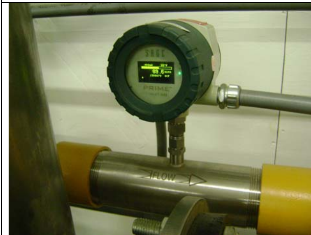
Sage Prim gas meter; gas to engine
