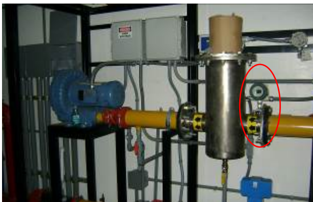
Engine gas flow meter (after dewatering and blower)
