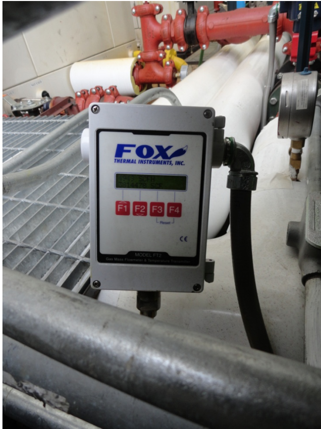
Natural Gas Meter
