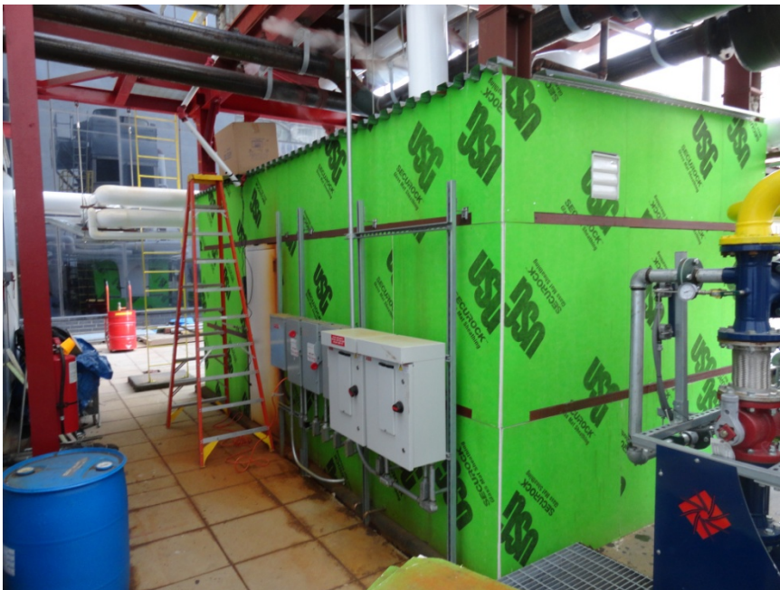
Hot Water Abs Chiller
