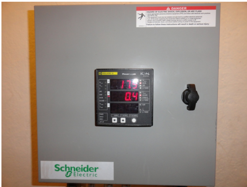
Parasitic Power Transducer – Located in Pump Skid
