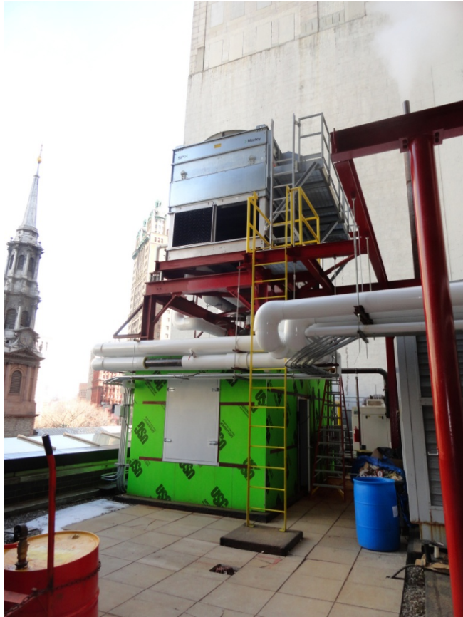
Hot Water Abs Chiller and Cooling Tower
