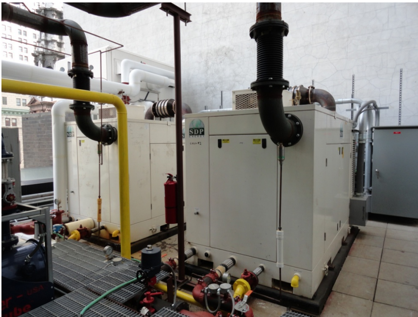
SDP 250 kW CHP Engine Generators
