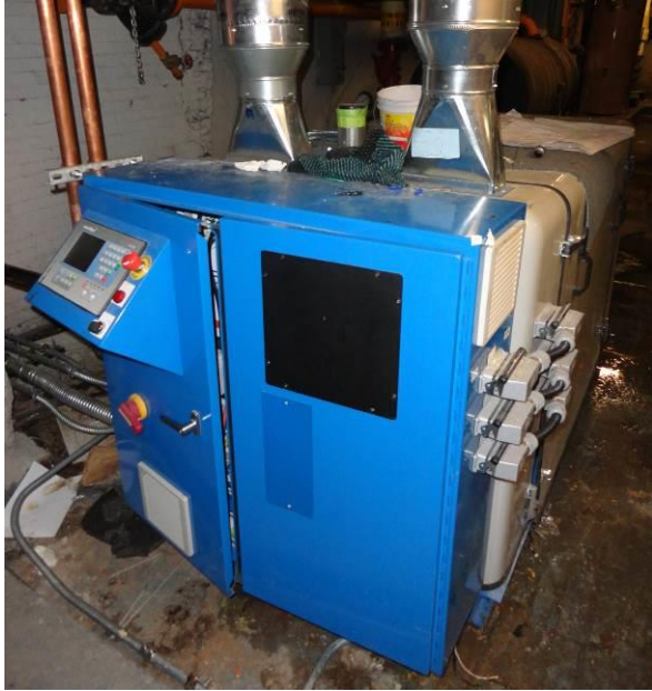
One of two (2) installed cogen units.
