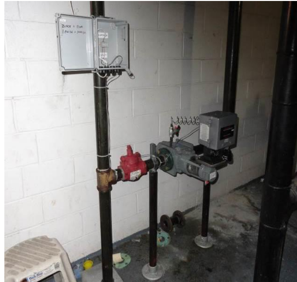
Utility provided gas meter and demarcation point.
