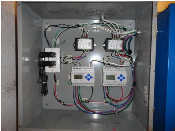
Total facility power meters (WT1, WT2)
