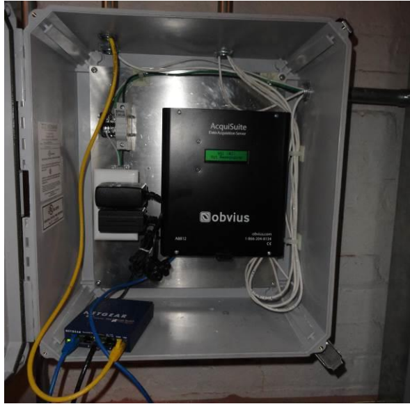
CDH datalogger and enclosure.
