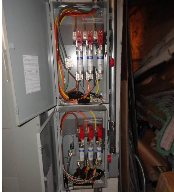
Power meters for generator #1 and generator #2 (WG1, WG2)
