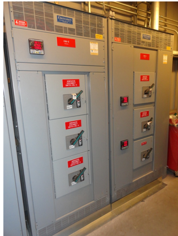
Generator #3, #4, & #5 Disconnects (Middle) Generator #6 Disconnect (Right Top) Generator #7 Disconnect (Right Middle)
