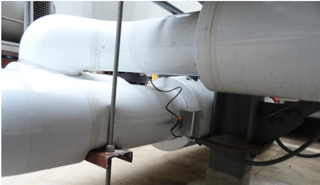
CHP Return Temperature From Useful HXs – TLR1
