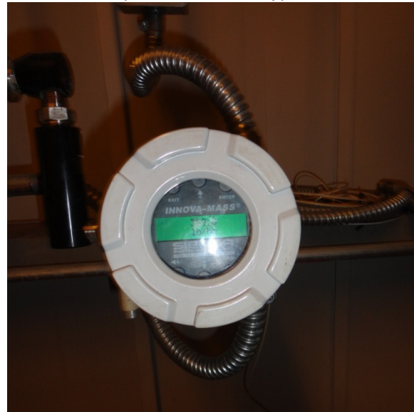
Steam Flow Reading – 369 PPH
