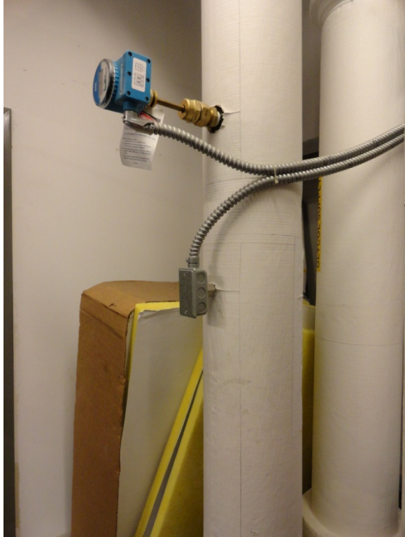
CHP Loop Flowmeter - FL Figure 11. CHP Loop Flow Sensors
