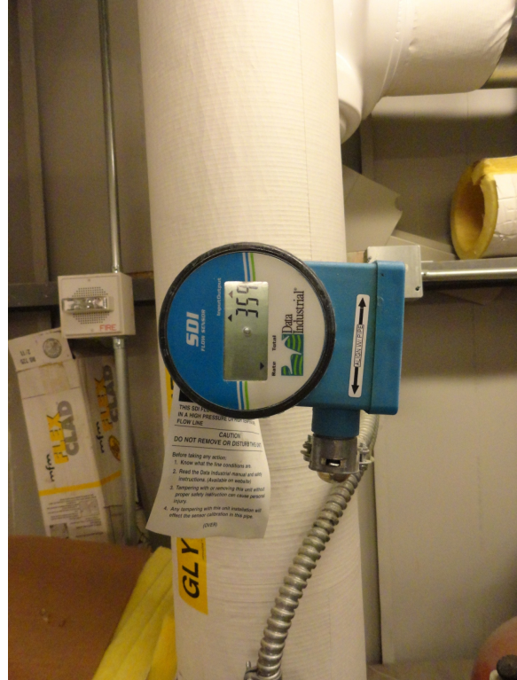
CHP Loop Flowmeter – Reading 359 GPM
