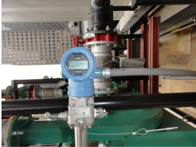
Figure 14. DP Gas Meter at CHP Skid (Not used for M&V)
