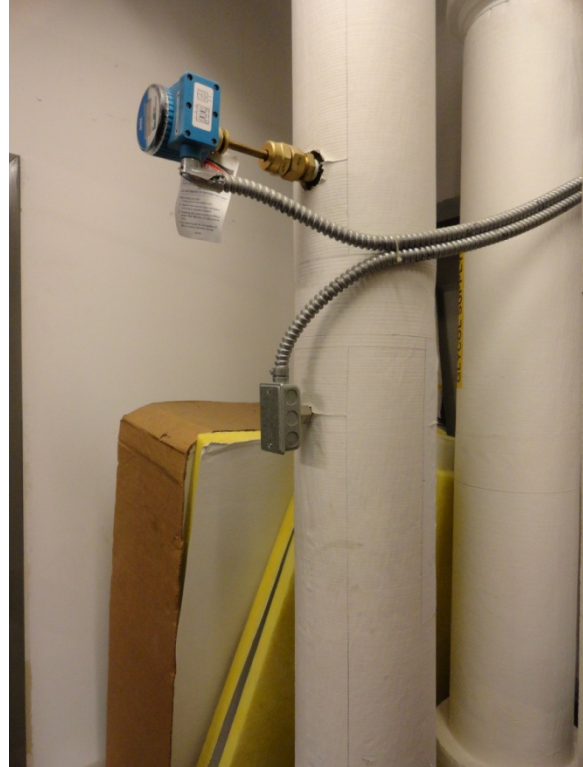
CHP Supply Return from Dump HX Temperature and Loop Flow – TLR2 & FL
